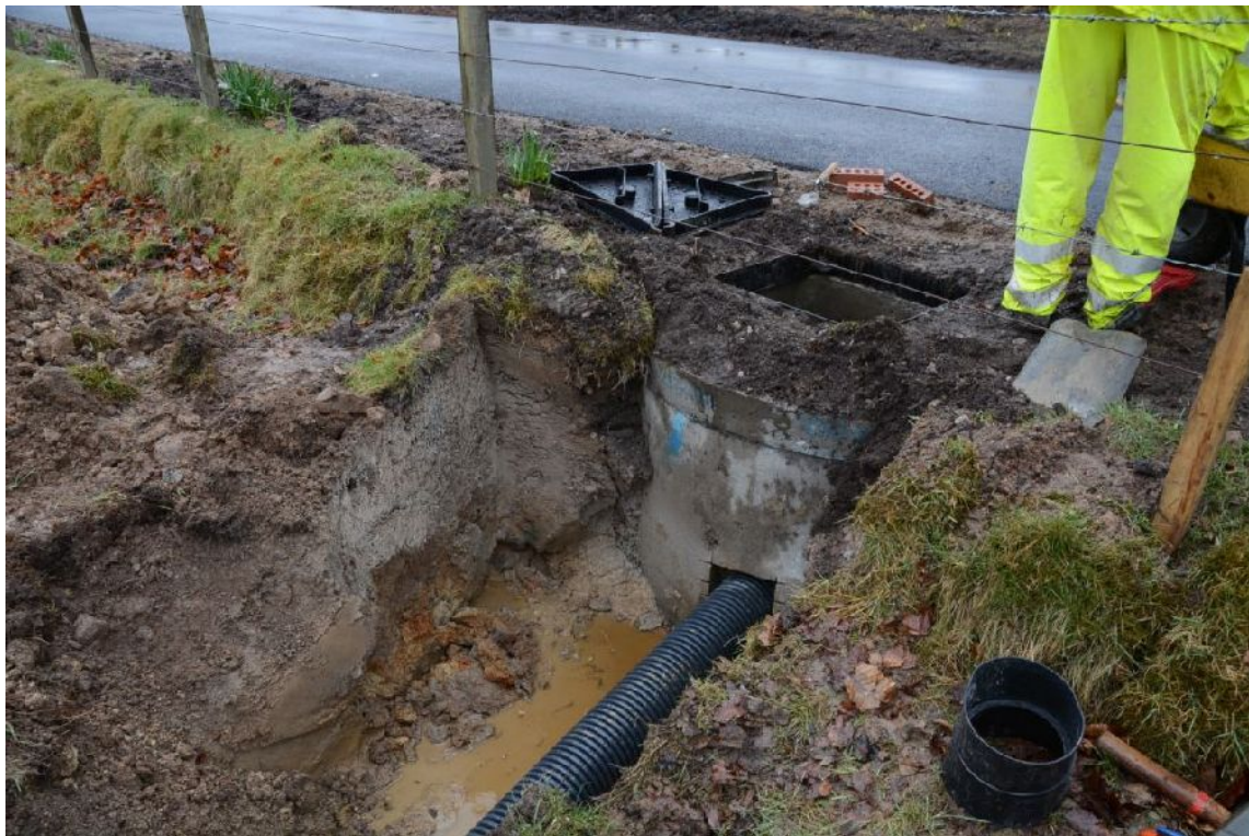
Illus 4 Silt trap in drain trench 1 with outlet to drain trench 2 into field
