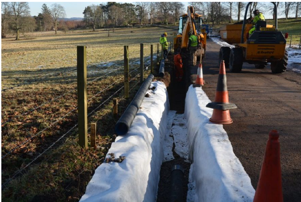
Illus 2 Drain trench lined with geotextile. Plastic pipe and gravel filled in.
