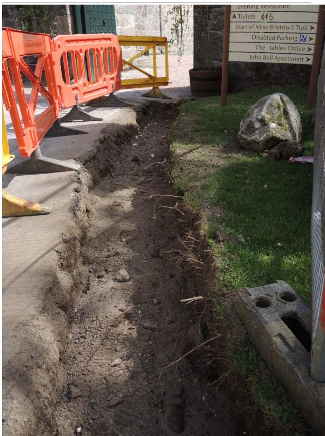
Illus 16 Gully running to W side of archway
