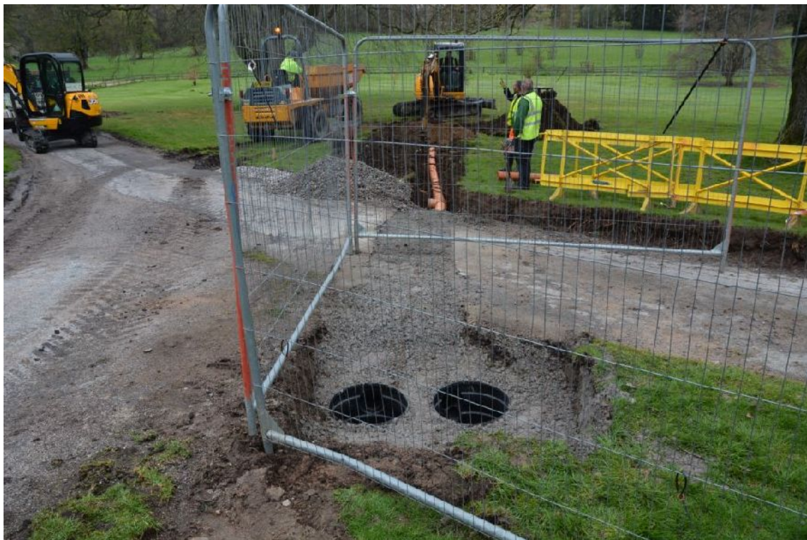
Illus 14 Drain from triangle to soakaway in grass to W of castle
