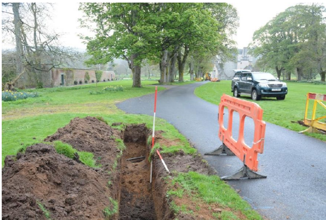
Illus 12 Grip 23 showing shallow topsoil. Water pipes (F) across S end of trench.
