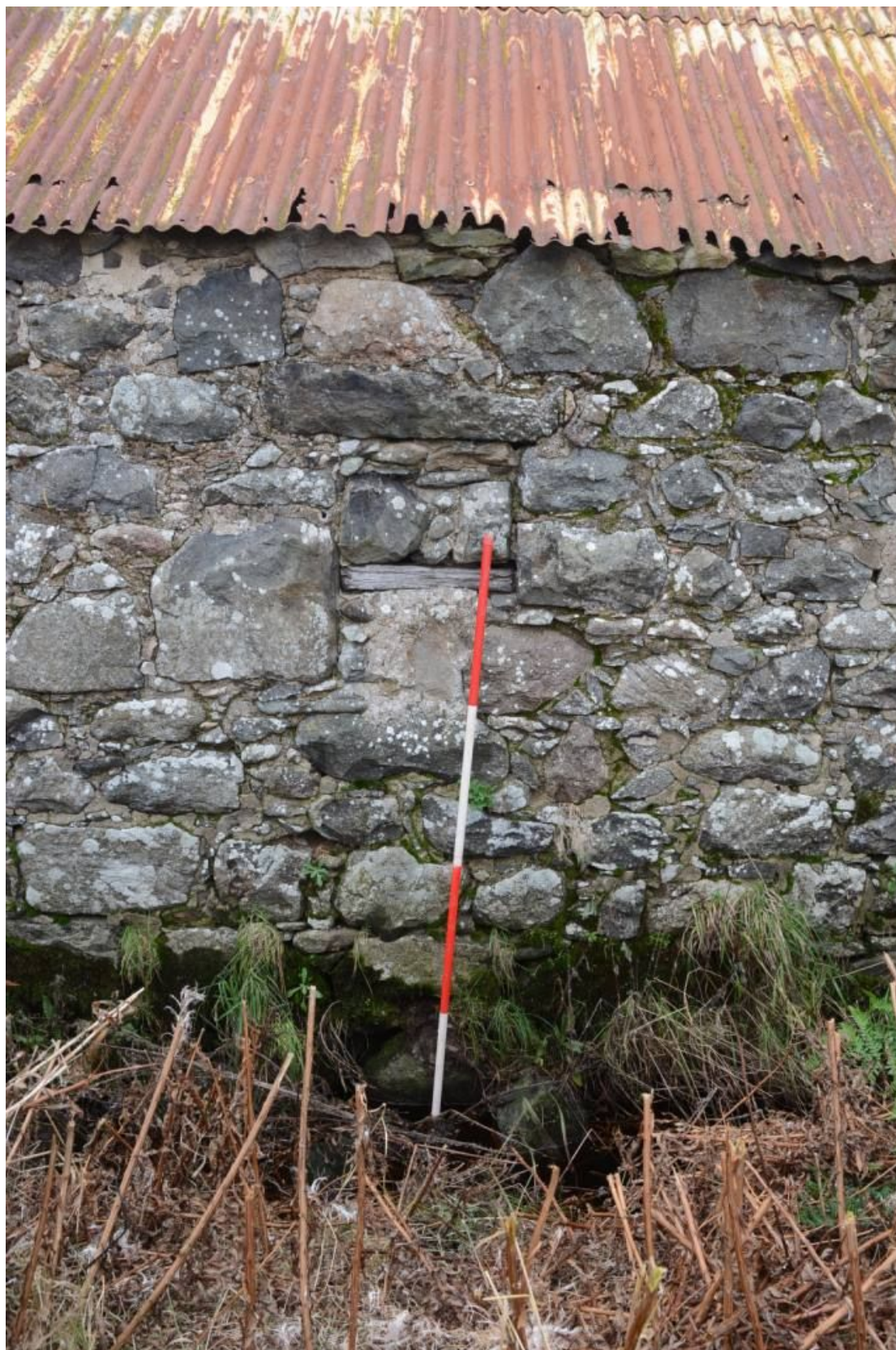
Illus 8 S wall. Blocking F3. The lade runs along the base of the wall.
