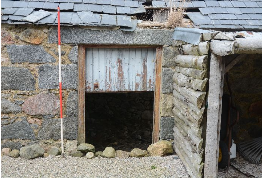
Illus 7 Wall 2. D2. Note dark grey lintel and stonework
