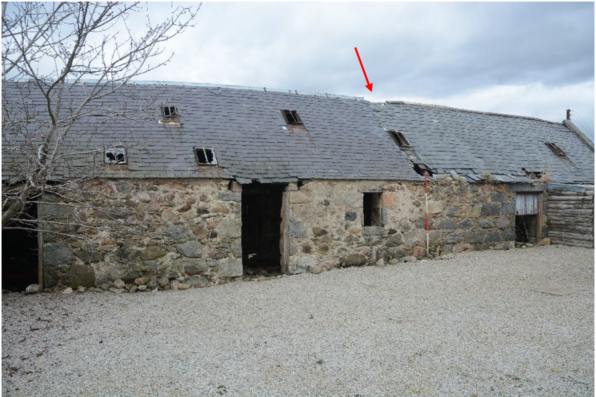
Illus 6 N Range. . Wall 2. The ranging rod indicates the difference between the roof and wall materials of the E and W ends of the structure (marked by arrow)
