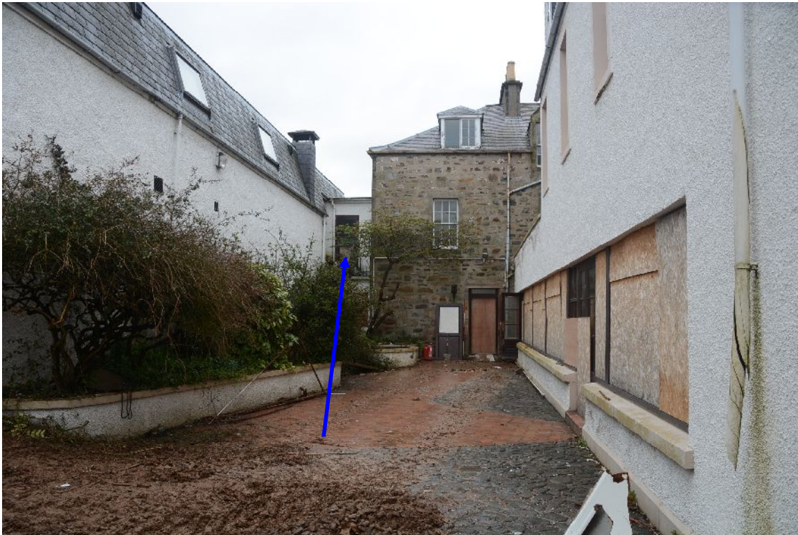
Illus 14 External view of wall NW of wing to be demolished. . Blue arrow marks position of pend in original building.
