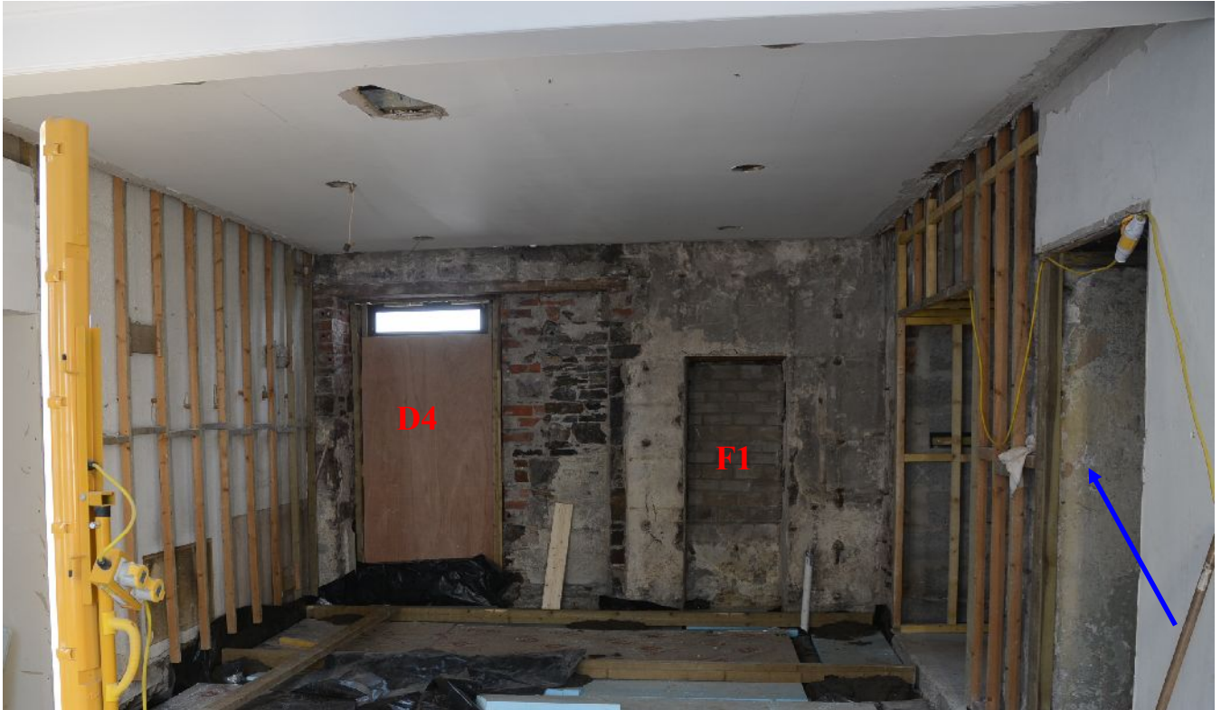
Illus 15 Detail of wall NW of wing to be demolished. Blue arrow marks position of pend in original building.
