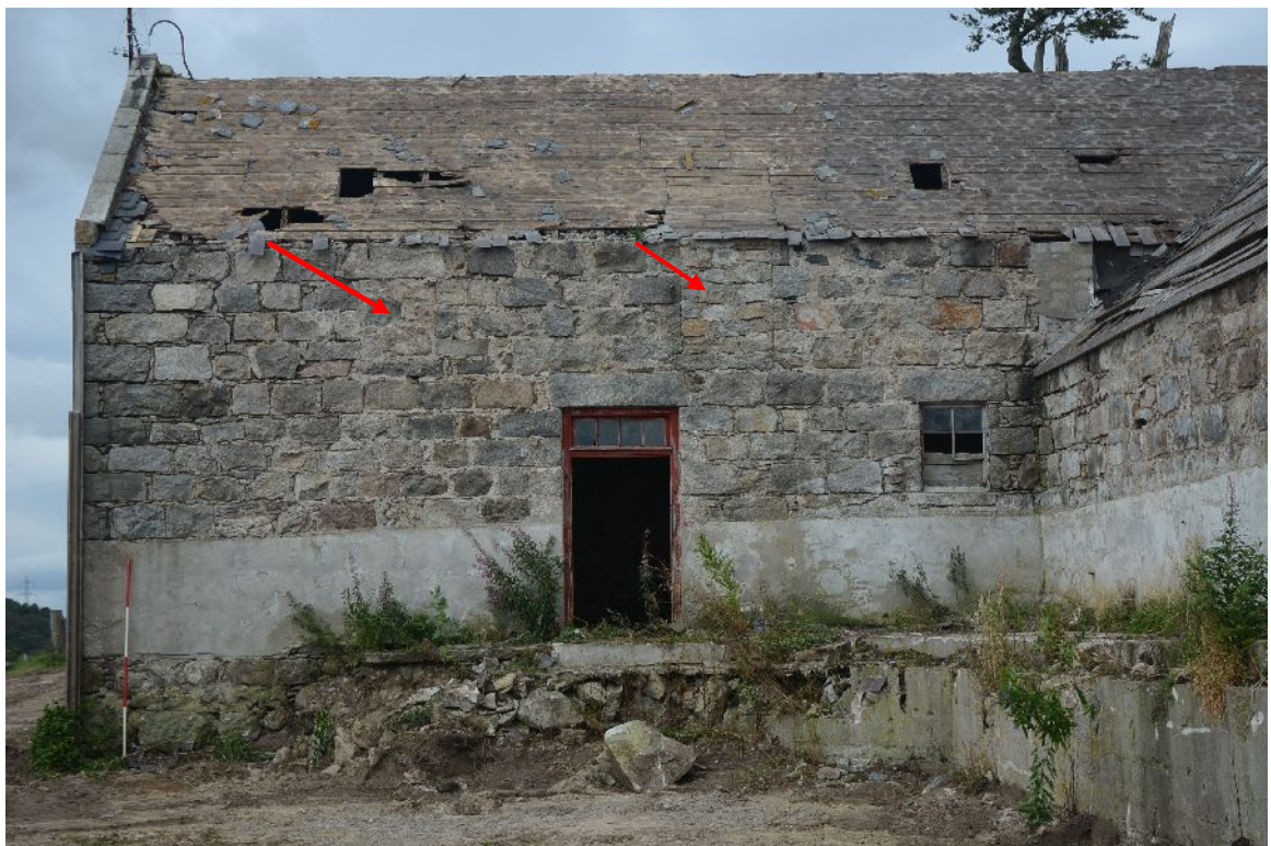
Illus 13 Building 1. Wall 4. E elevation of W Range. Note blockings W3 & W4 (arrows)
