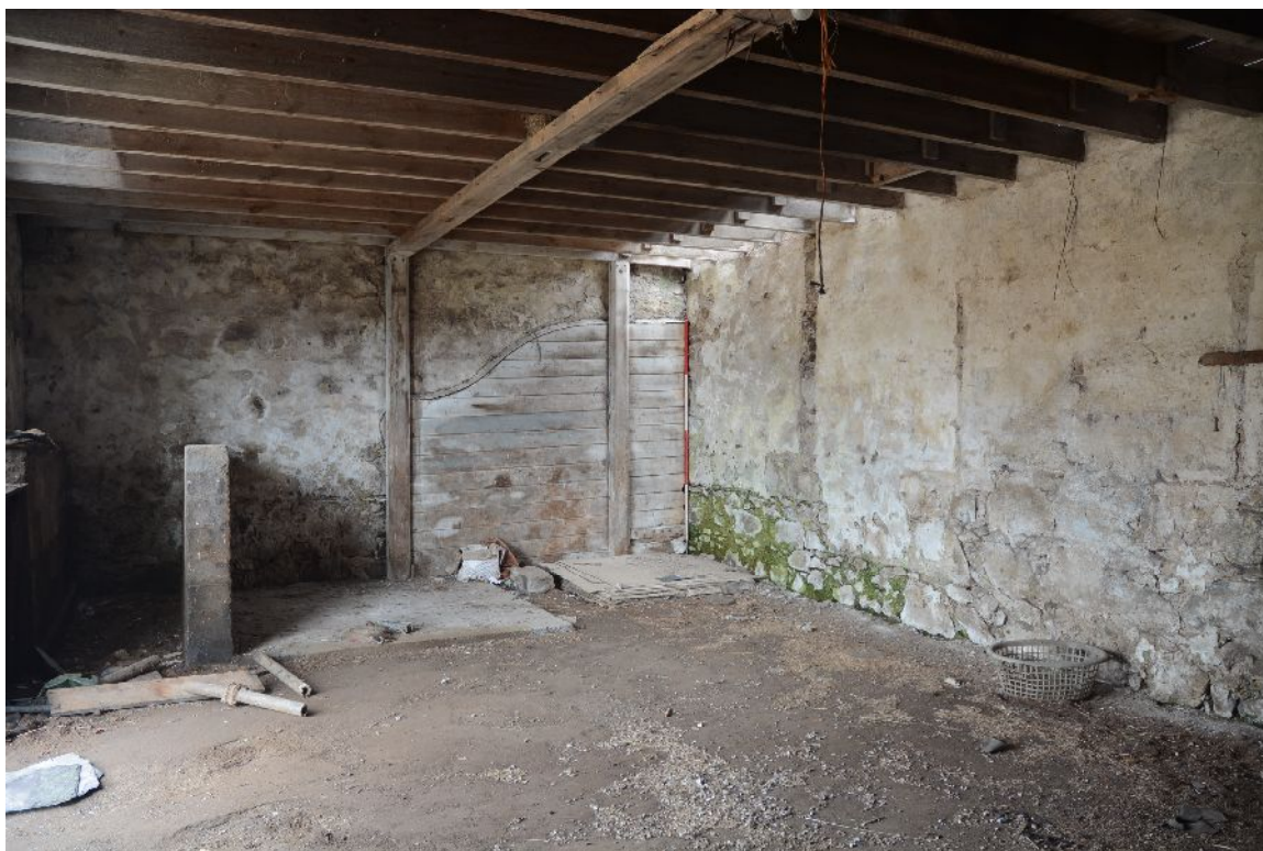
Illus 36 Building 3. Trevis in N wall and trevis scars on back (E) wall
