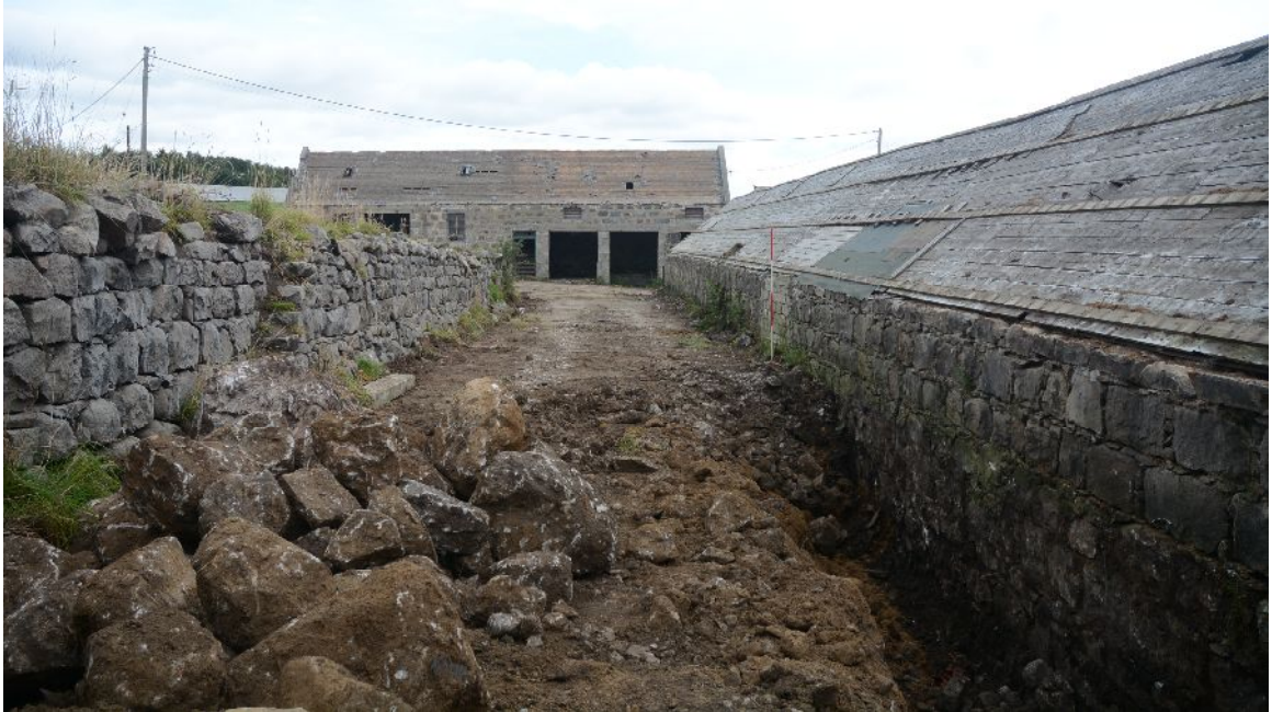
Illus 8 Building 1 N wall of N range . Blocked door D13 visible by ranging rod. Retaining wall to slope on LHS. Building 3 in background
