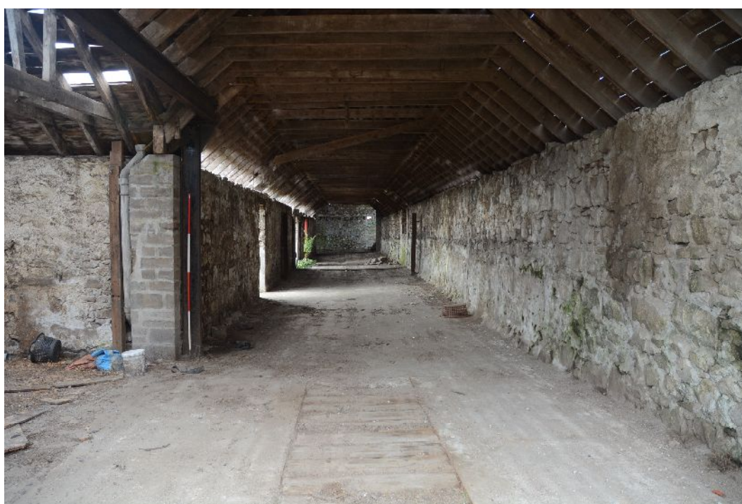
Illus 17 Building 1. Interior of N range looking W. Inspection pit in foreground.
