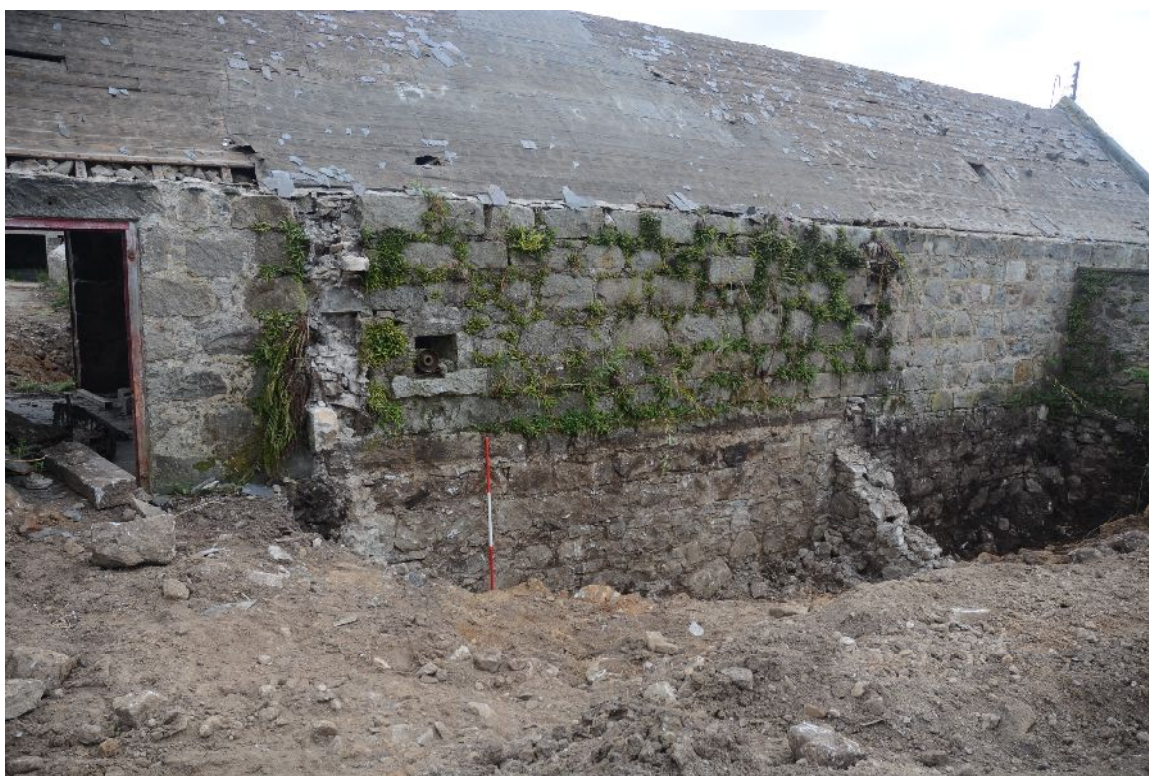
Illus 23 W wall (wall 6) of Building 1 with scar of Building B1b and shaft of F1 (above ranging rod)
