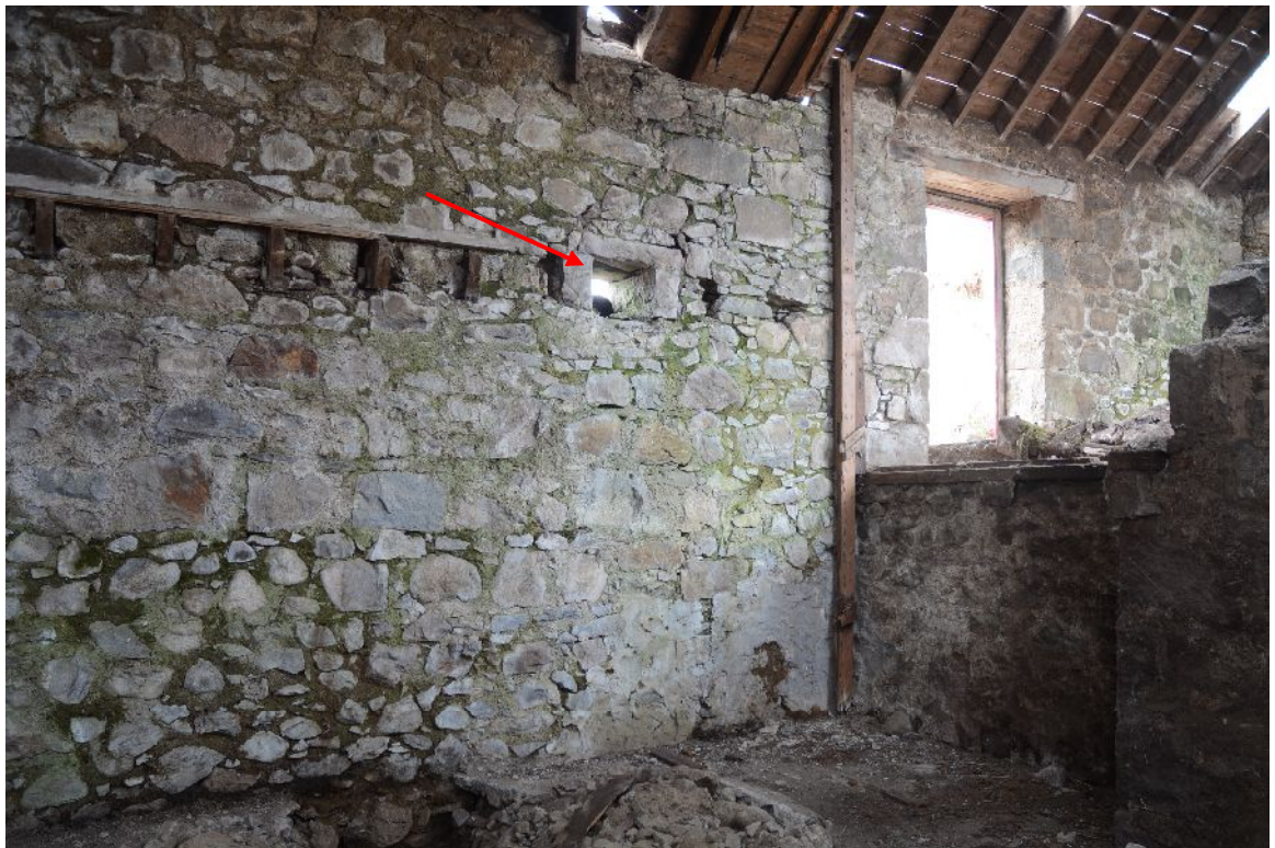
Illus 14 Building 1. F1 in W wall at level of loft floor.
