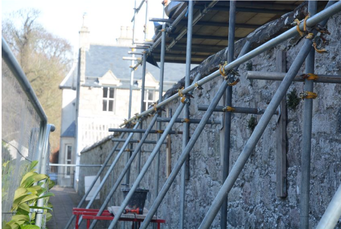
Illus 8 View along the W face of the W wall, looking towards the house. 2016 during remedial work on the wall
