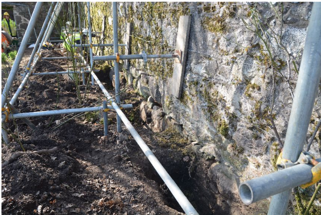
Illus 10 Inner face of W wall looking S, showing wedges placed in cracks before wall straightened
