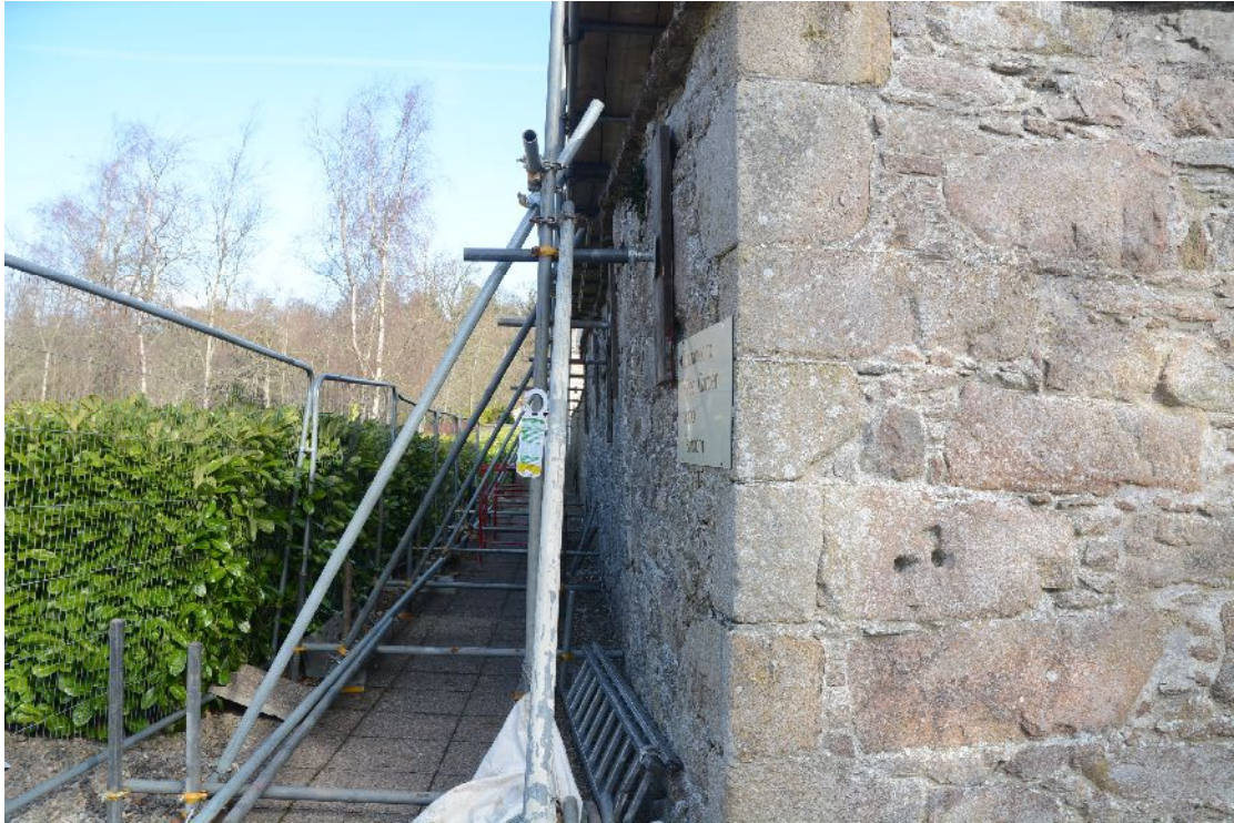
Illus 9 W wall looking N from SW corner showing bulges
