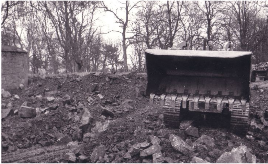
Illus 6 Major earthworks removing the drystone dyke 1961 (NTS archive photo 0366 from HLS)
