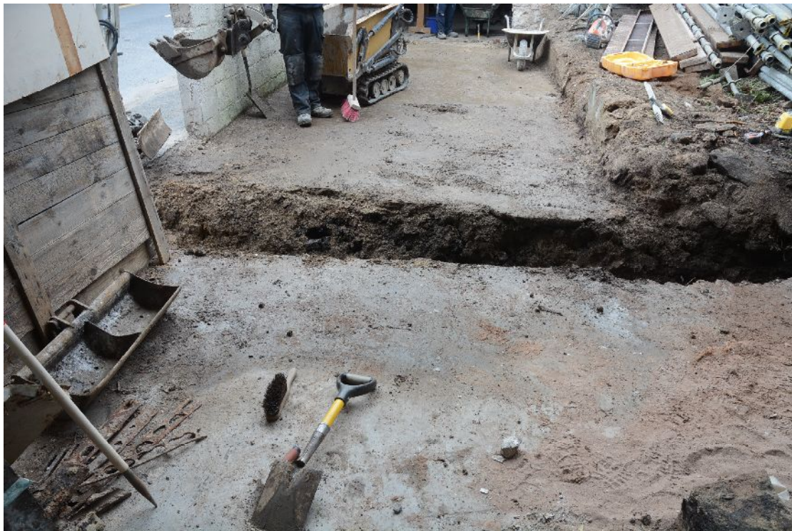
Illus 4 Looking N from No 8 George Street across the trench on the line of the removed N gable
