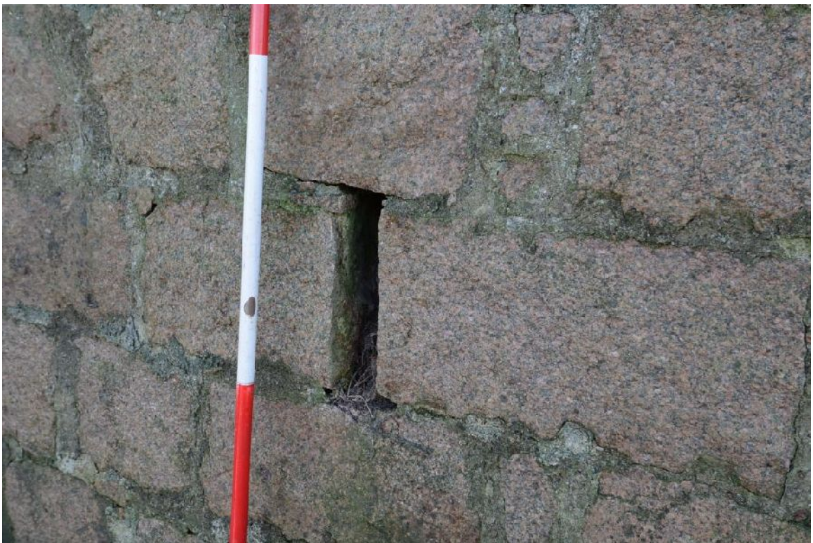
Illus 13 Building 1. Blocked vent F1
