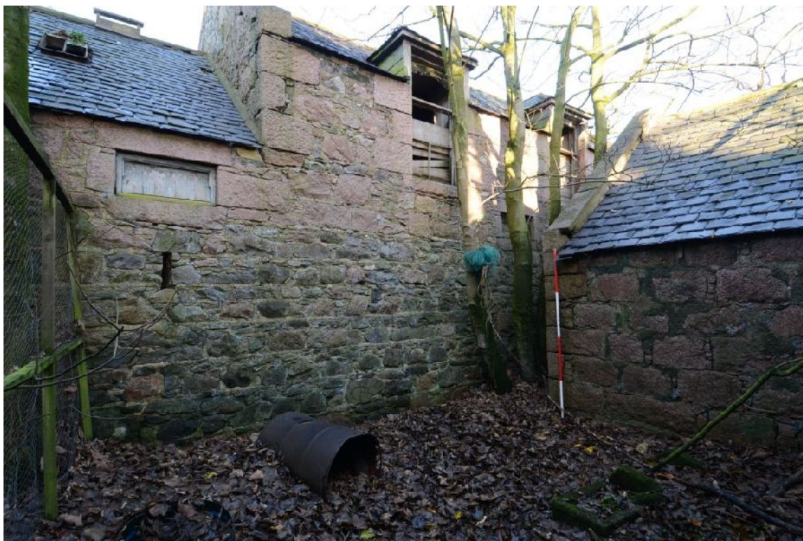
Illus 24 Building 2 (RHS) in relation to back of S range of steading. Note slit vent comparable to blocked vent in Building 1
