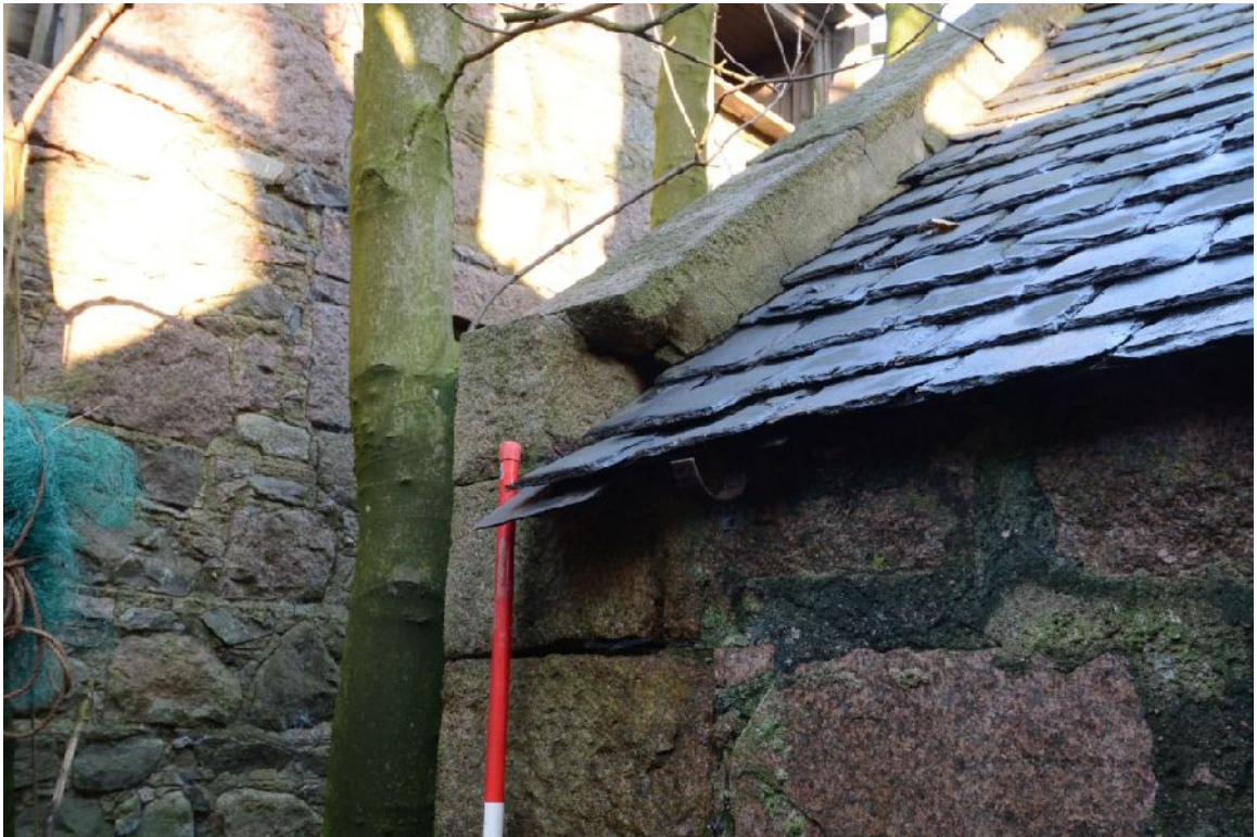
Illus 14 Building 2 NW corner showing skew and skewputt
