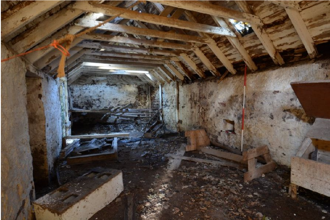
Illus 18 Building 2, Area E, looking NW to possible stable. Door D6 on LHS foreground. Alcove F2 beside ranging rod.
