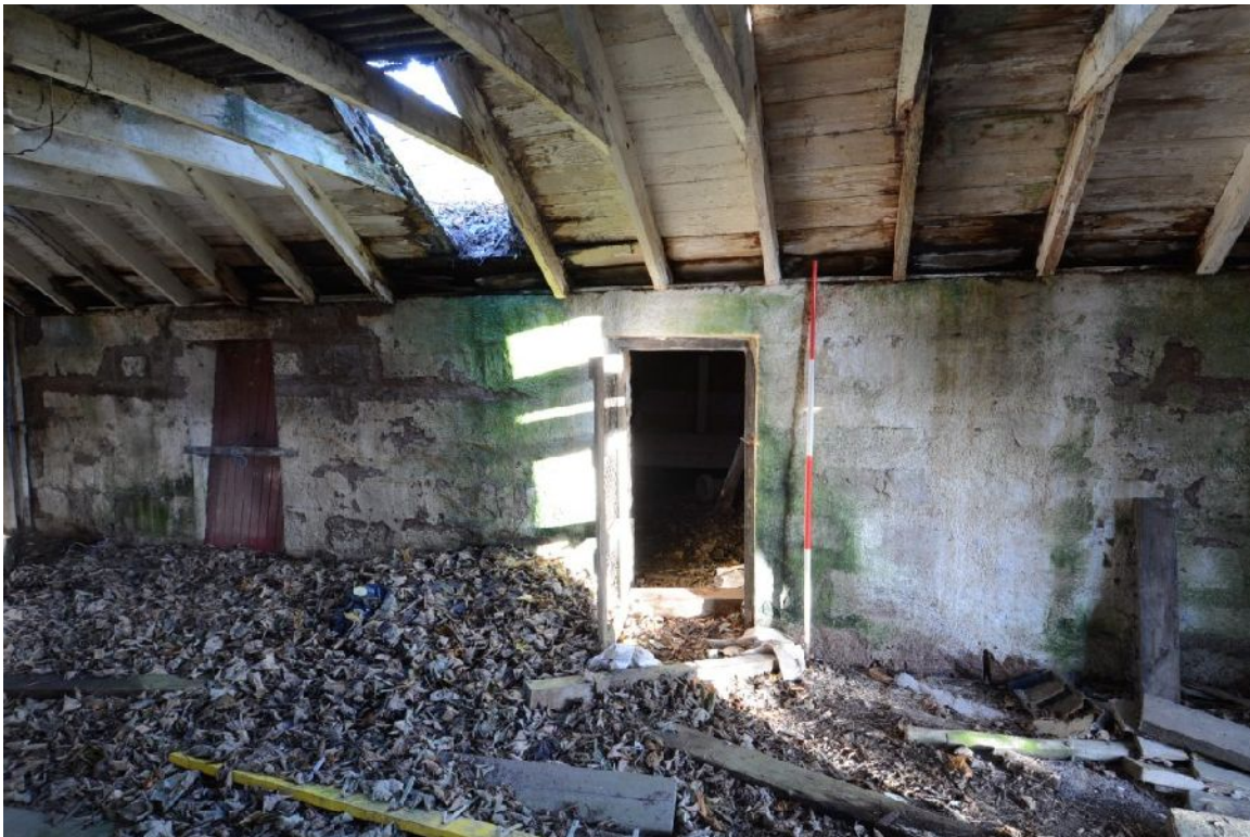
Illus 17 Original outer wall of Building 2 seen from inside Building 3. Ranging rod stands beside door D5
