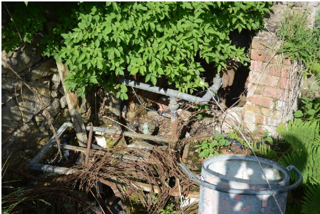
Illus 99 Pipe work in lower floor area at E end of Boiler House 25
