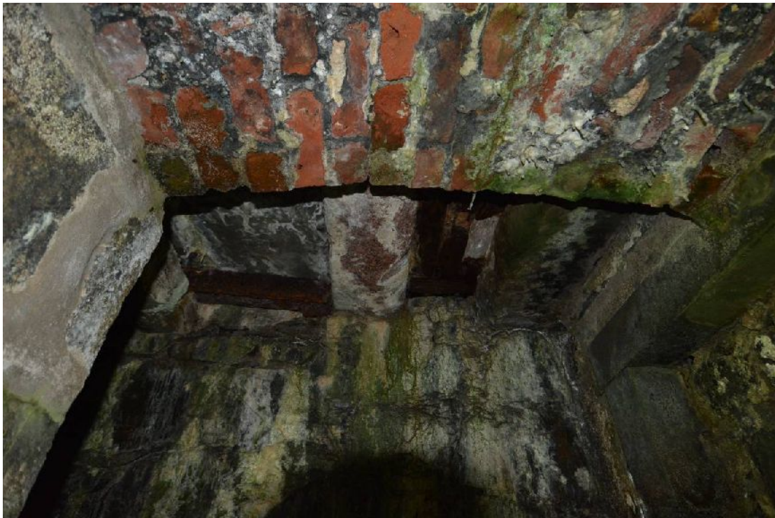
Illus 74 Roof of chamber below steps. Blocked door into garden house visible on RHS
