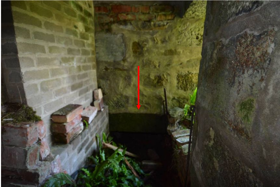
Illus 73 Arrow shows channel below steps
