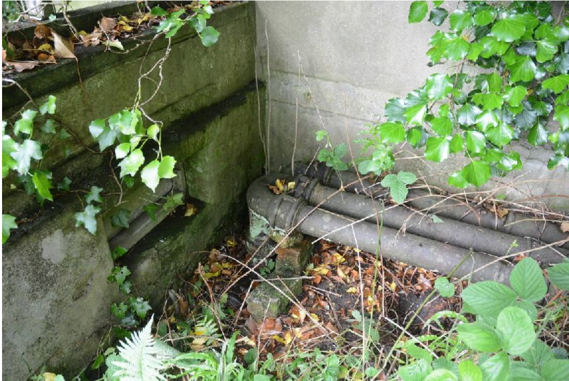
Illus 93 Greenhouse 28. Heating pipes and scar on back wall indicating height of staging
