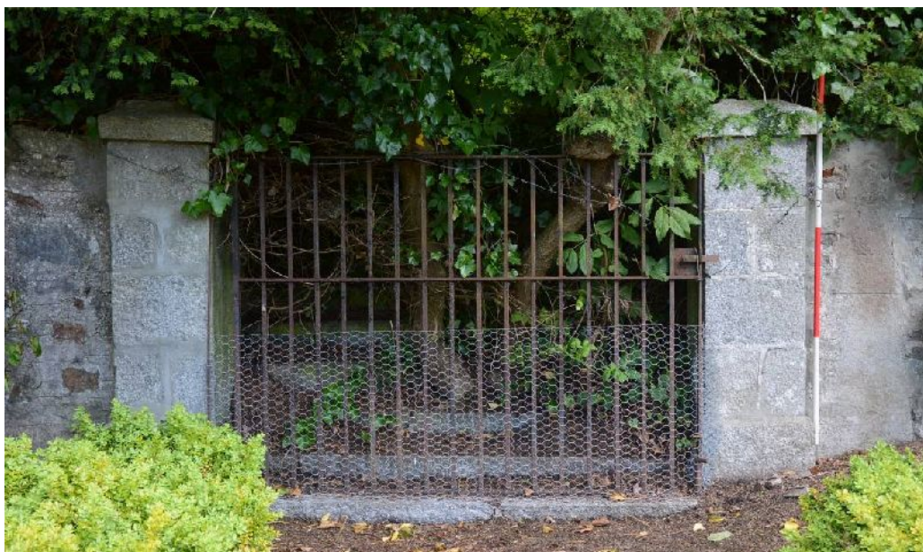
Illus 44 Gate 21 internally from walled garden to lower terrace of new castle
