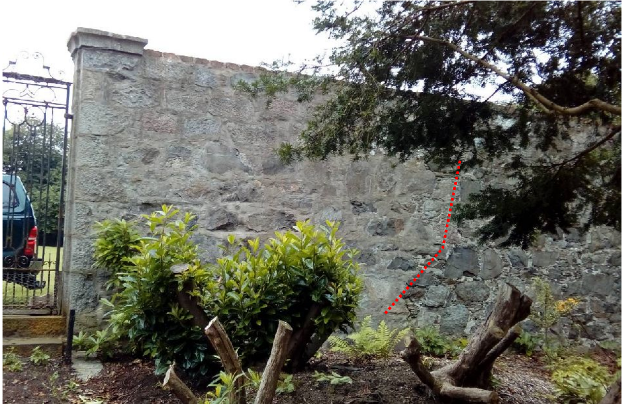
Illus 25 S wall W of central gate. Red line indicates break in construction
