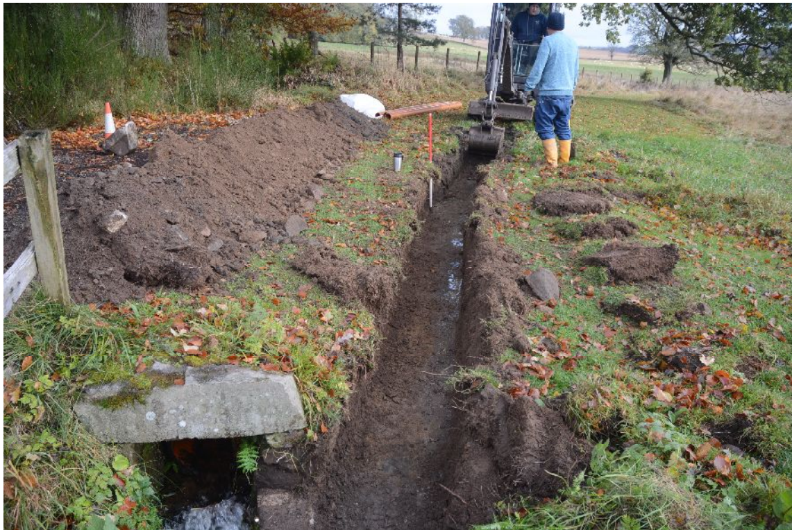
Illus 13 Drain looking E. Electric cable at base of trench beside ranging rod
