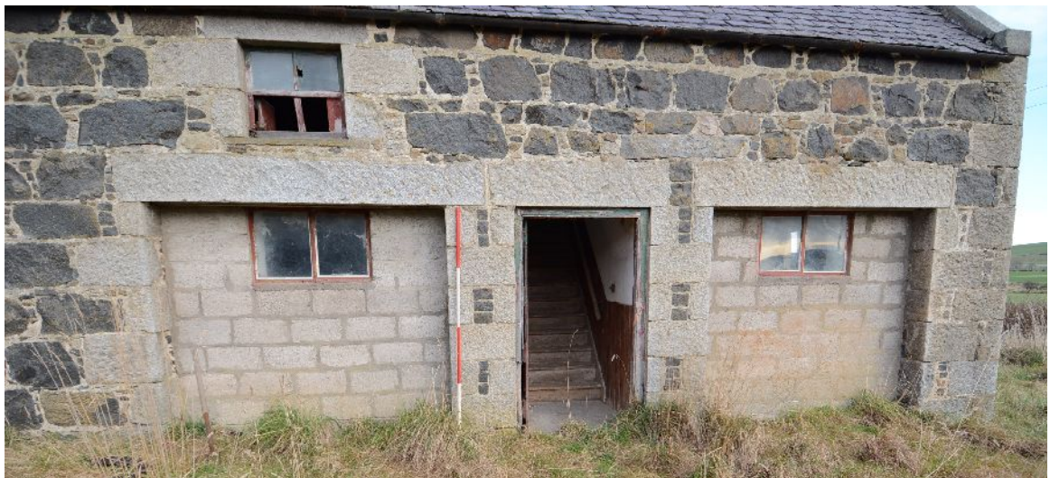
Illus 15 Detail of blocked cart bays D11, D13 and door to loft D12
