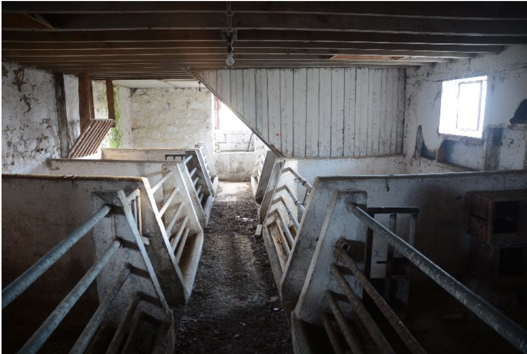
Illus 25 Area F cart bays converted to piggery. Note base of loft stair
