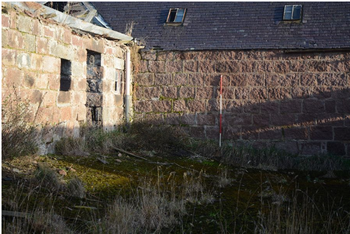
Illus 21 Inside court, junction of N range and E range, showing difference in stonework
