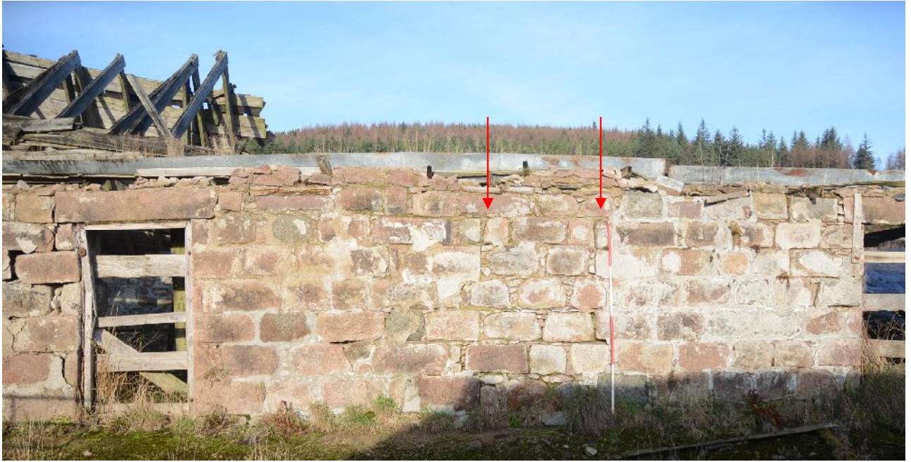
Illus 10 S wall of N range, between doors D4 and D5. Blocking F1 marked by red arrows.
