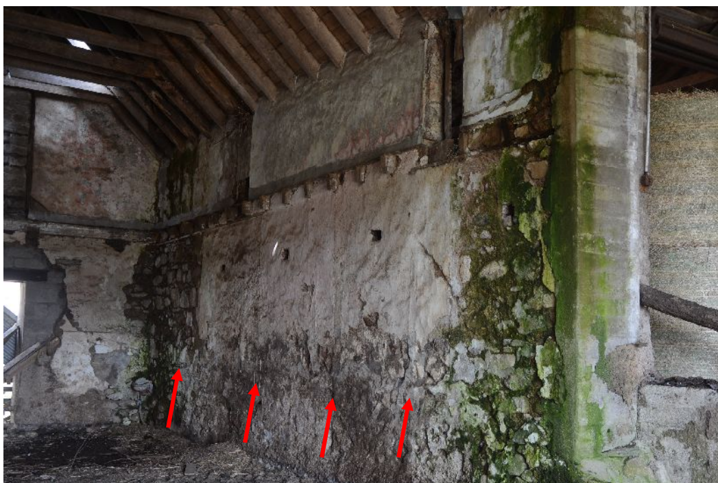
Illus 16 Interior of Building A looking W along N wall. Note joists of loft floor. Arrows mark trevis scars. Modern break-through to Building B on RHS
