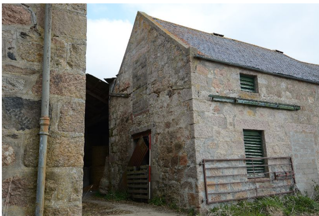
Illus 18 W gable of Building A showing blocked door to hay loft.
