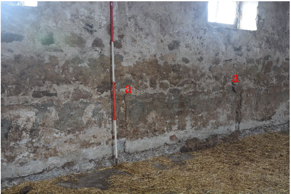
Illus 27 Detail of interior S wall of Building G with scars of original tied cow stalls (a)
