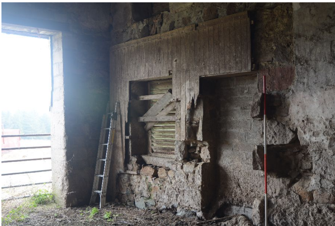
Illus 15 Pine paneling inside S wall art E end of Building A. Ranging rod indicates remains of cross-wall.
