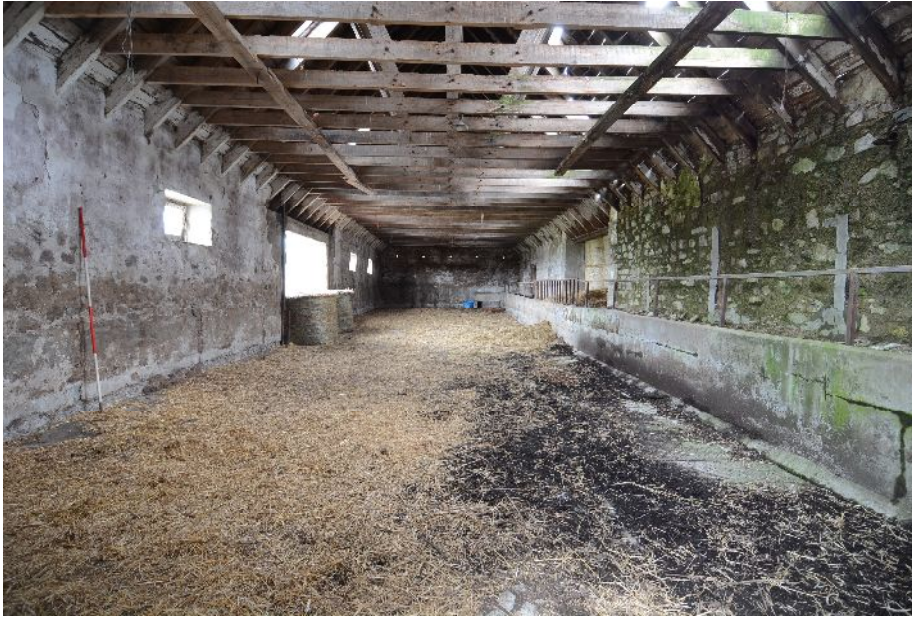
Illus 26 Building G looking W. Feed pass on RHS. Ranging rod beside scar of tied cow stall on LHS Interior Although converted into a modern open cattle building with a raised concrete feed pass along the N wall, scars on the inner face of the S wall suggest that it had originally been used for tied cattle with pens along the S ( and probably the N) wall.
