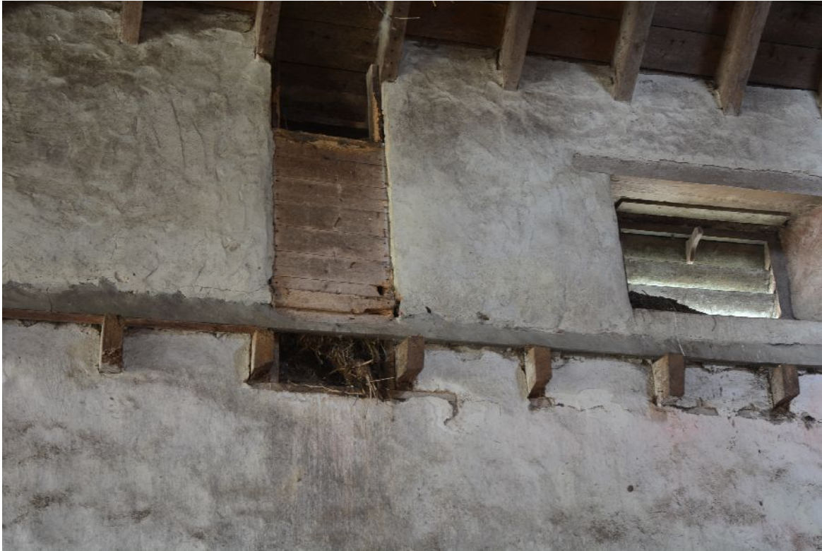
Illus 19 Inside S wall of building A showing chute from loft to stable
