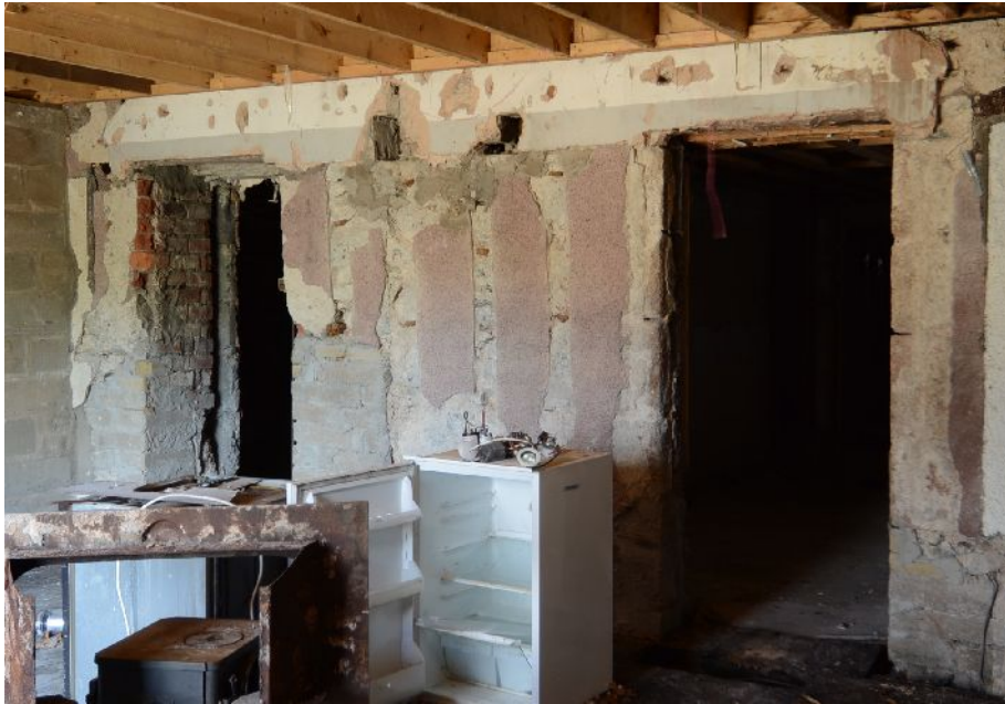
Illus 48 Doors D3 (LHS) and D4 (RHS) from inside the E single storey extension. Note stone rybats on D4 (Detail below)
