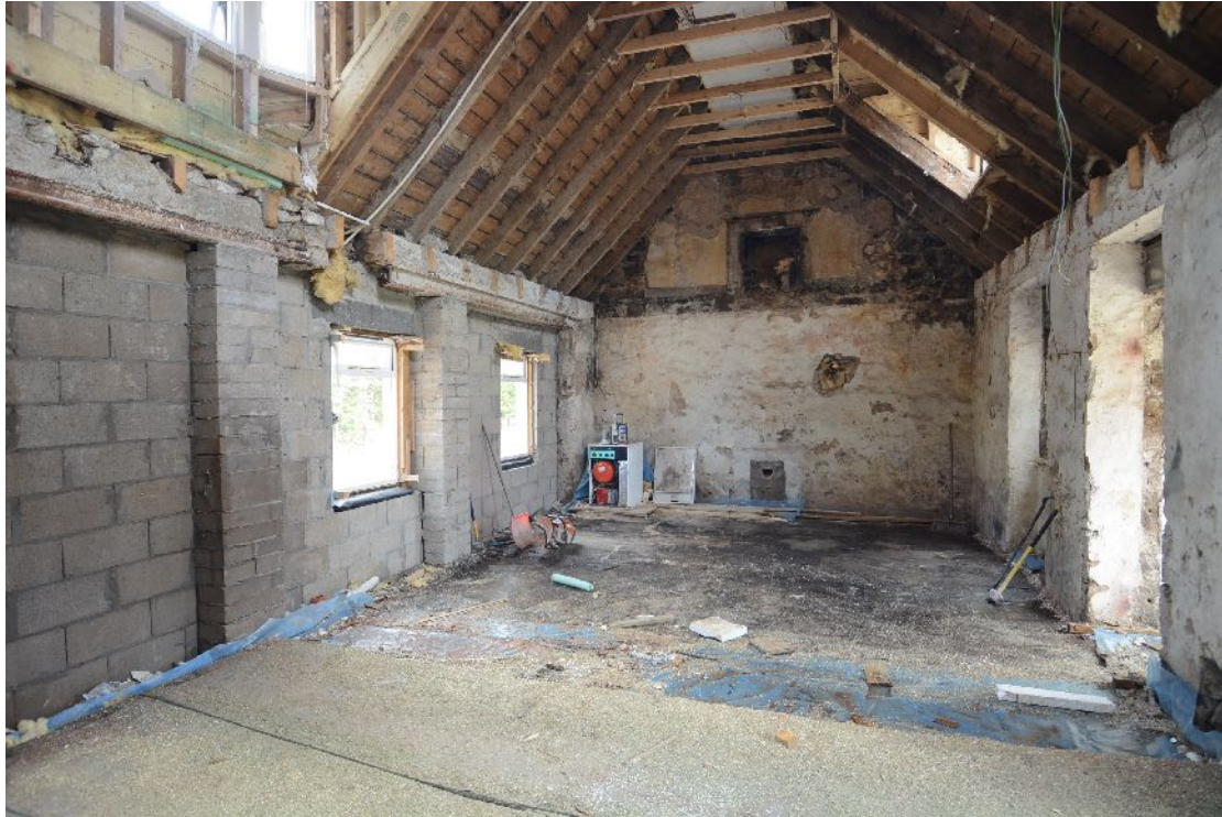
Illus 64 Interior of S house looking S with blocked cart/ carriage bay openings in front (E) wall
