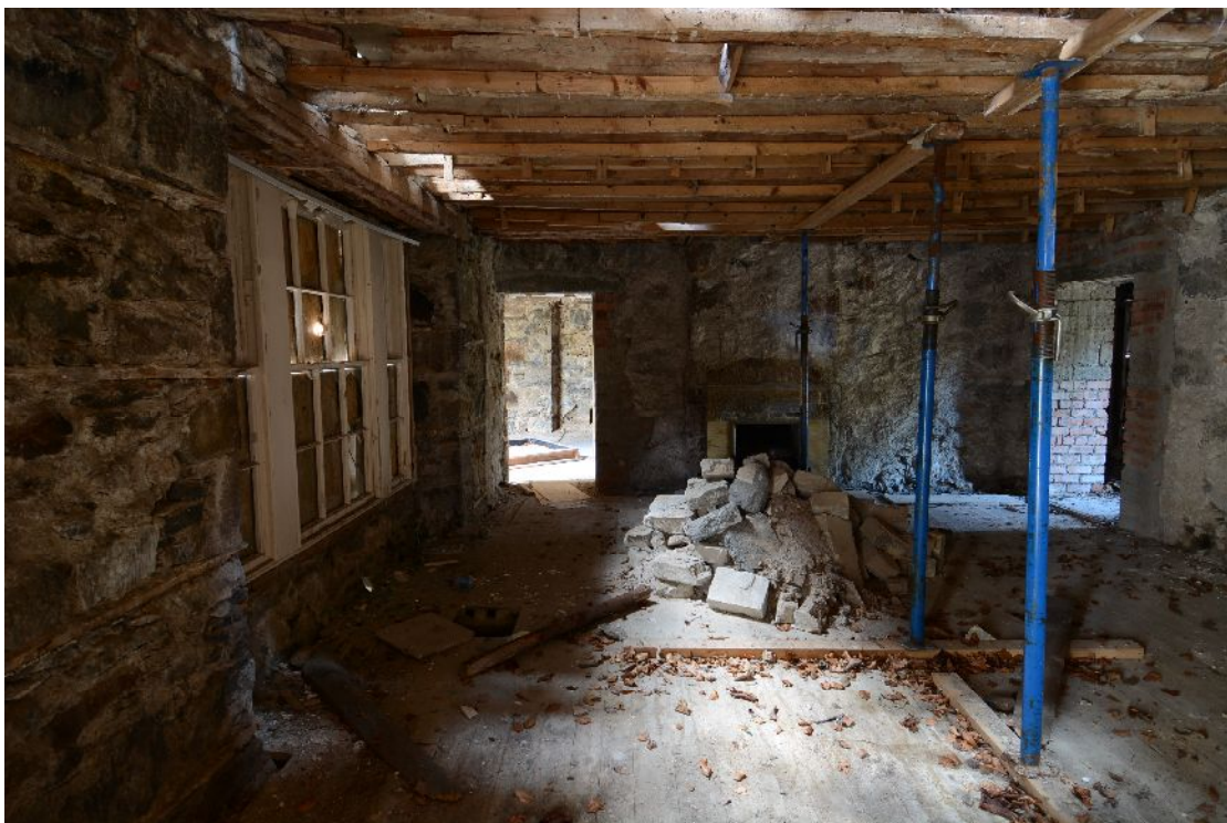
Illus 42 Room B looking W, fireplace F6 in background to RHS of door into Room C.
