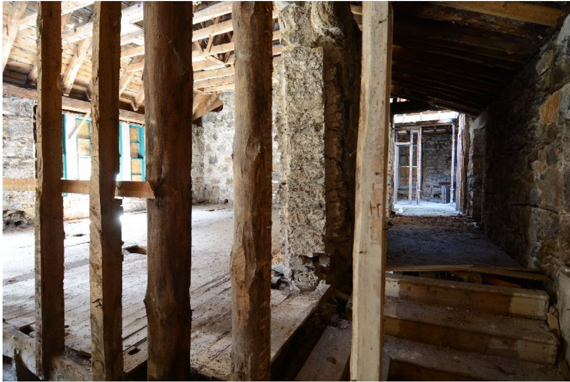
Illus 52 First floor looking S and W from top of main stair. To LHS is front centre room with fireplace on W wall ( above fireplace F6) . To RHS passage to rooms in W wing.
