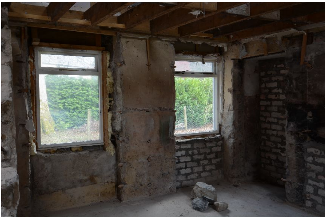
Illus 63 SE corner of N 'coach house' showing blocked door in front (E) wall and blocked door through to S 'coach house'
