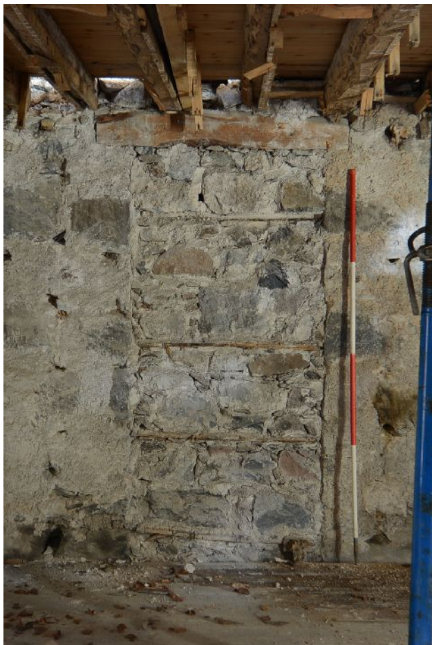
Illus 43 Room B. Doorways and blocked doorway F3 (RHS of ranging rod) in N wall. Detail of blocked door F3
