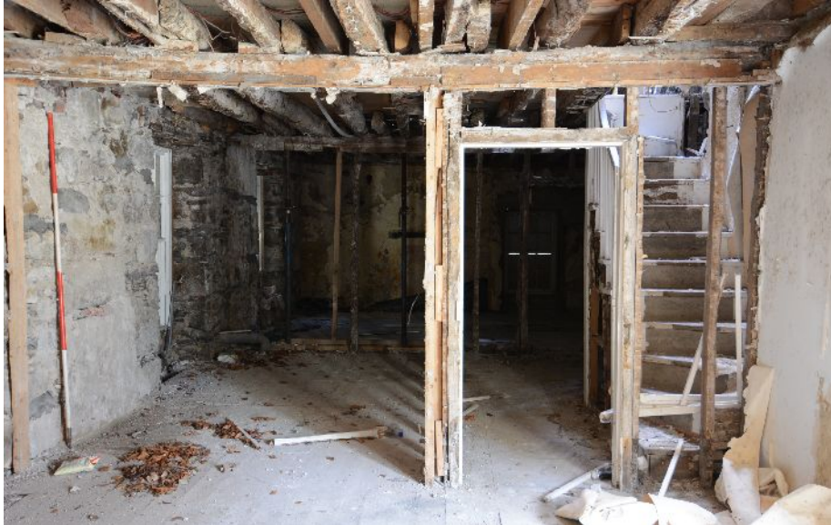
Illus 45 Room C looking N to Room D. Back stairs on RHS beside door into back passageway and back door to courtyard
