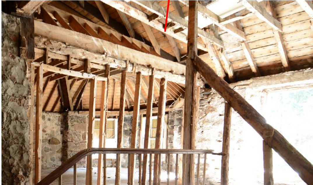
Illus 51 First floor room in E wing from top of main stair. In 1928 this was drawing room. Detail of roof timbers
