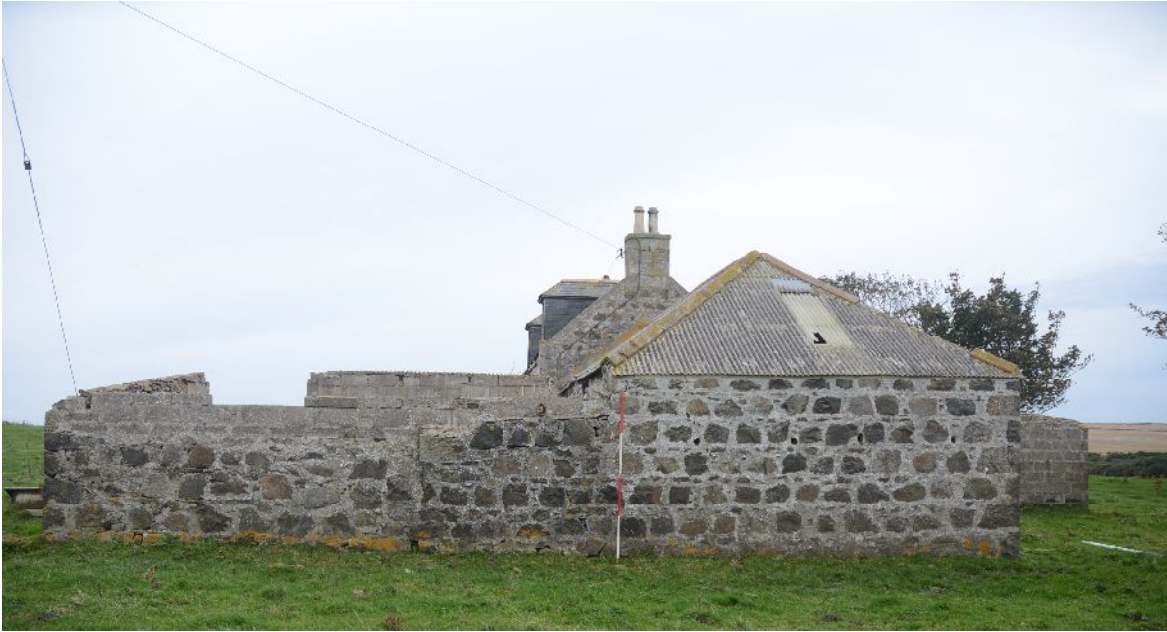
Illus 9 Building 2 from N with Building 6 abutting it on LHS beside ranging rod.
