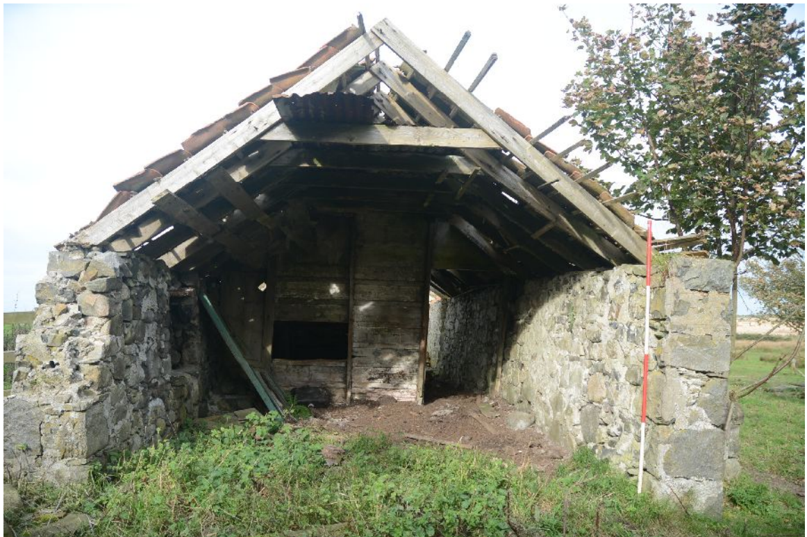
Illus 30 Building 3. S range S wall broken through.
