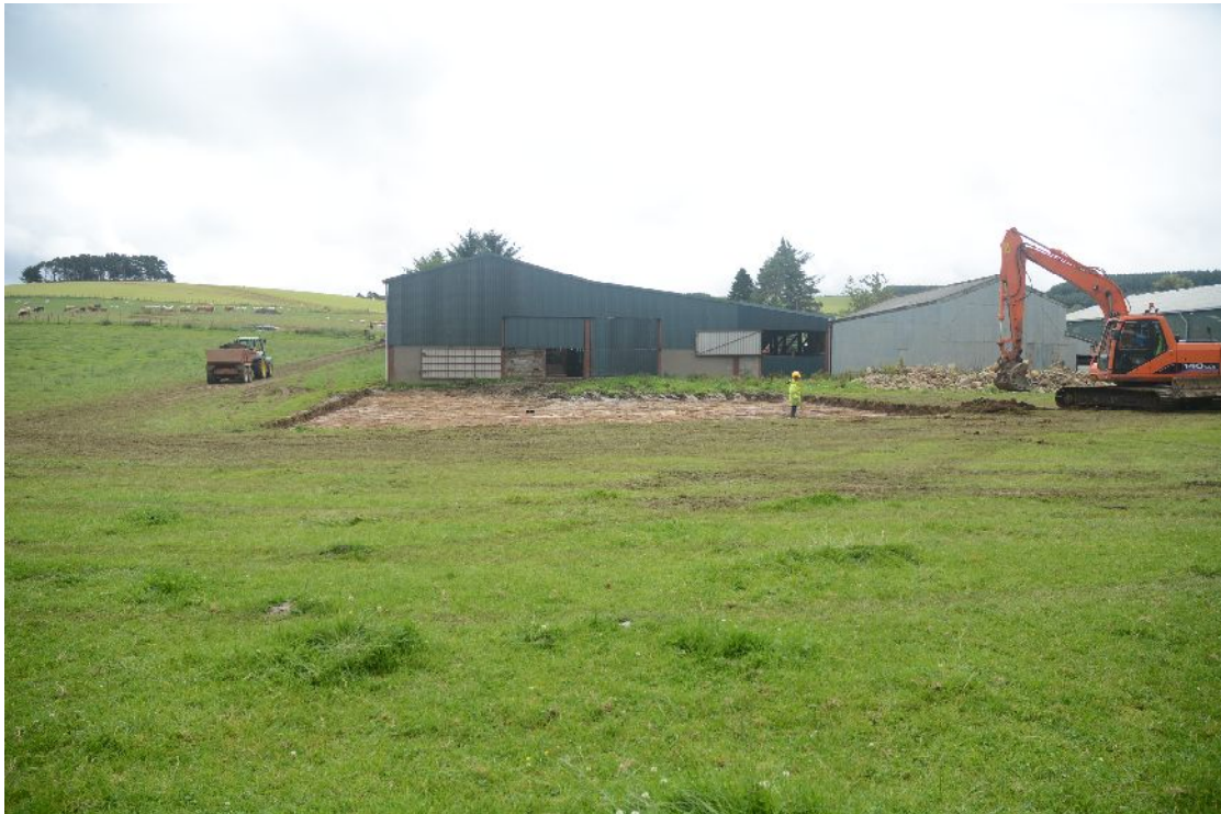
Illus 4 Looking S towards Hawk Hill (trees on top) showing site of new shed in relation to existing buildings.
