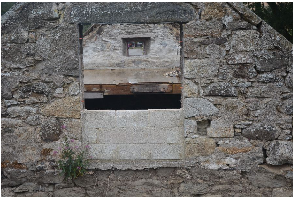
Illus 12 Window W1, looking through building to loft floor and window W2
