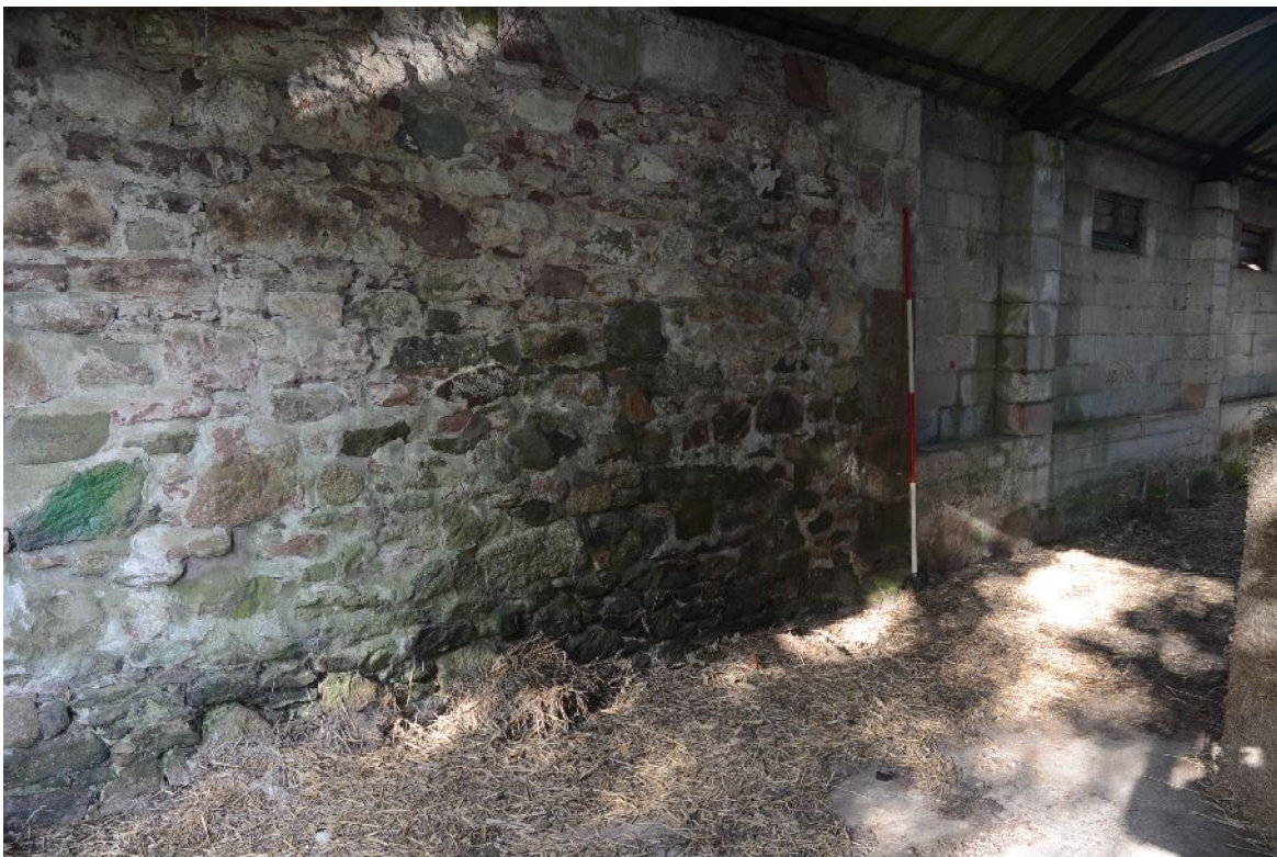
Illus 44 Building D. Inside of N wall with 19 th -century stone wall in foreground and at base of concrete wall
