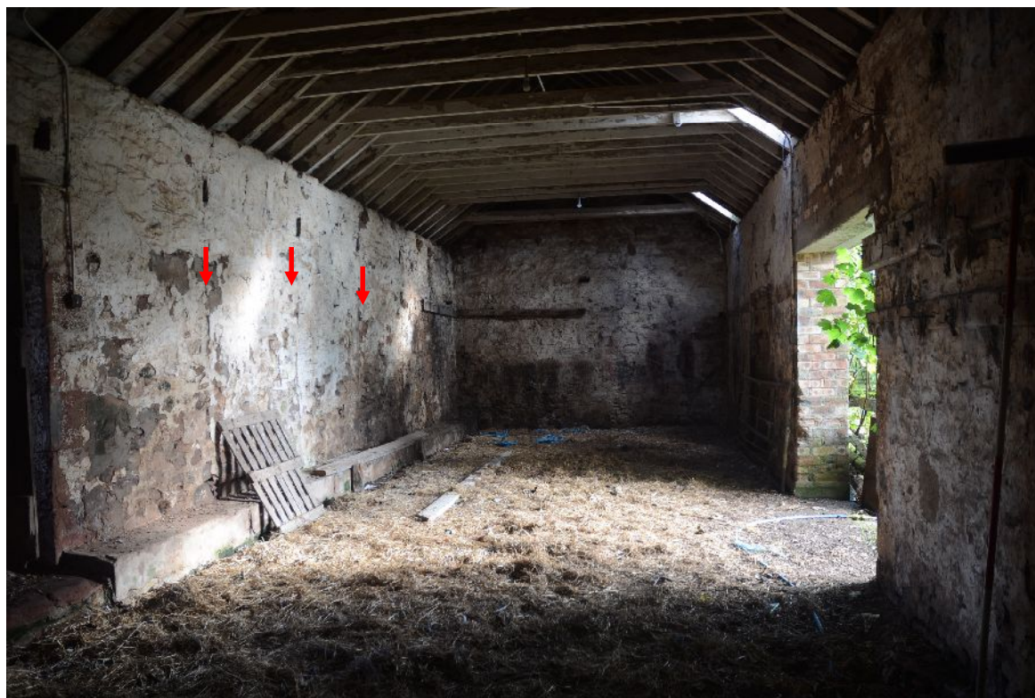
Illus 27 Building B looking S Red arrows indicate some of possible trevis scars
