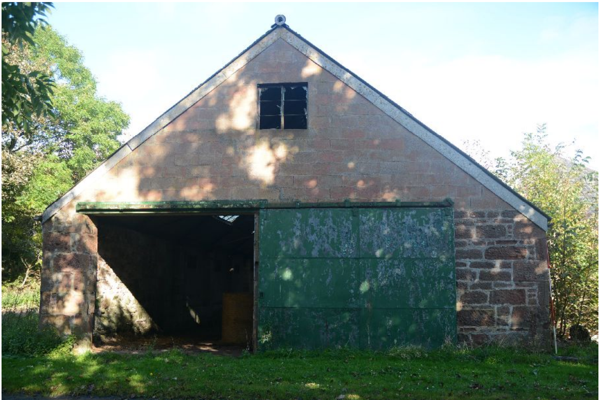
Illus 41 Building D. W gable with sandstone to wall head and concrete blockwork above. Door D19.
