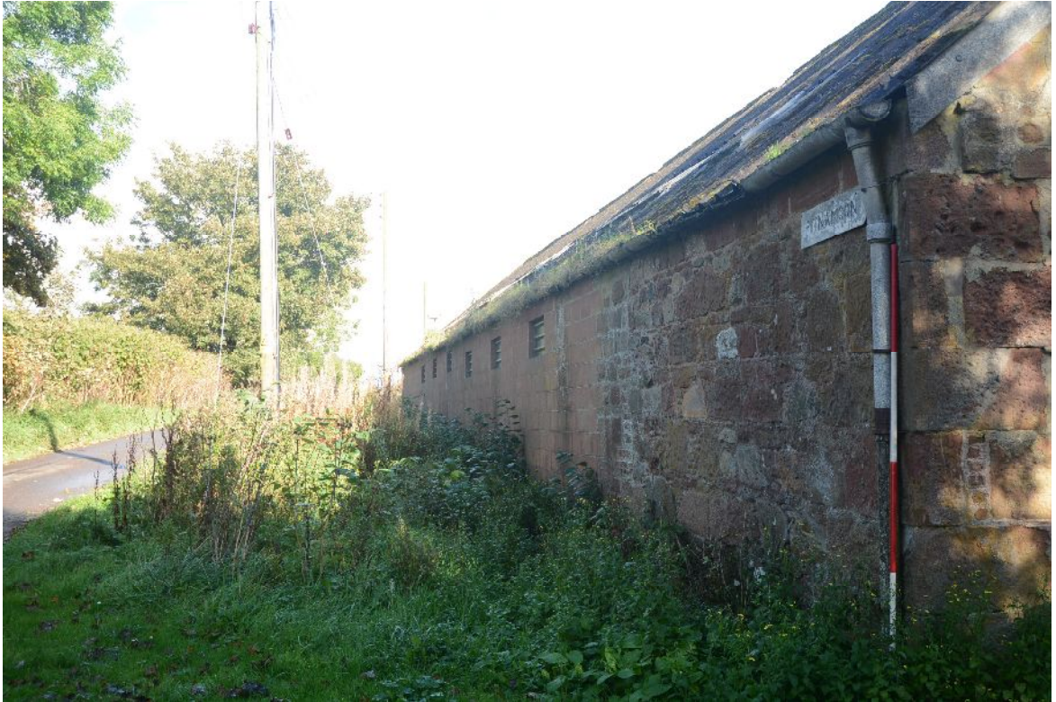
Illus 43 Building D. N wall, looking E. Stonework of 19 th C wall in foreground. Vents in concrete wall.
