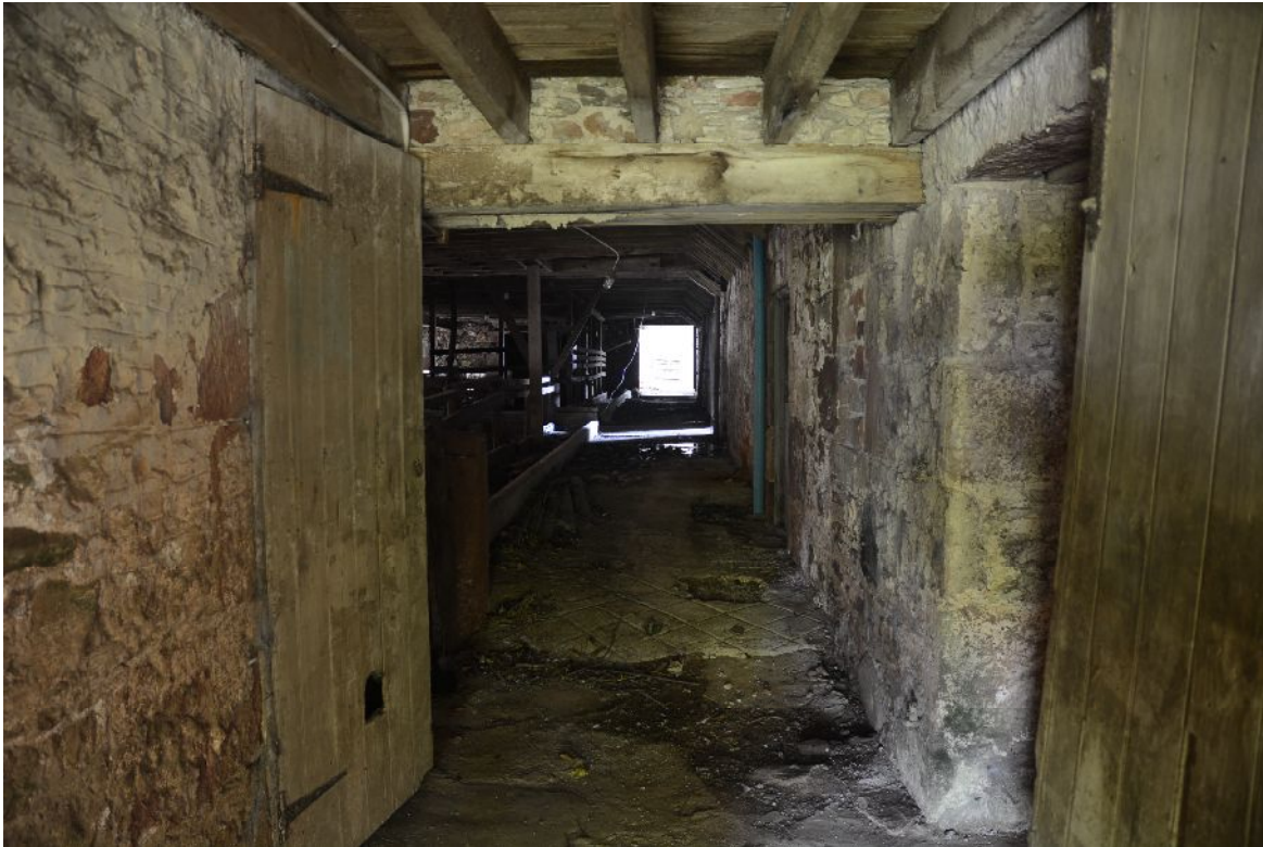
Illus 36 Looking N along W wall of Building C (RHS) from door D6
