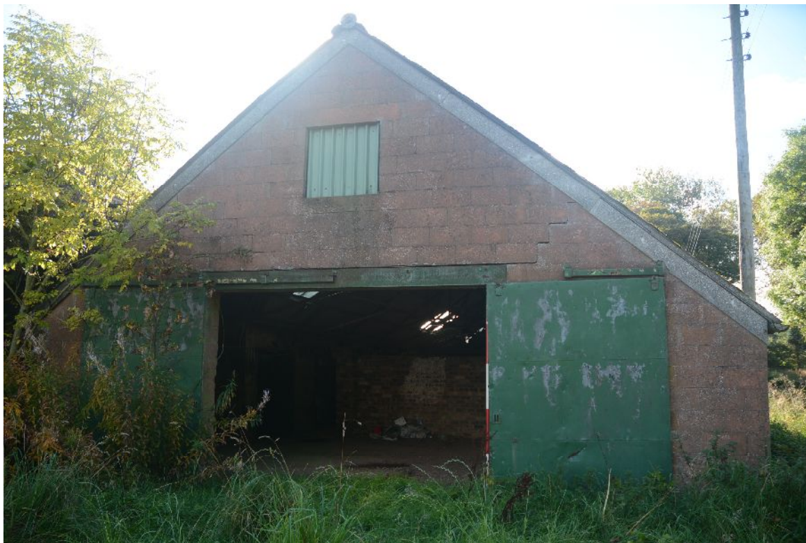
Illus 42 Building D. E gable with concrete block wall. Door D13 with vent above.
