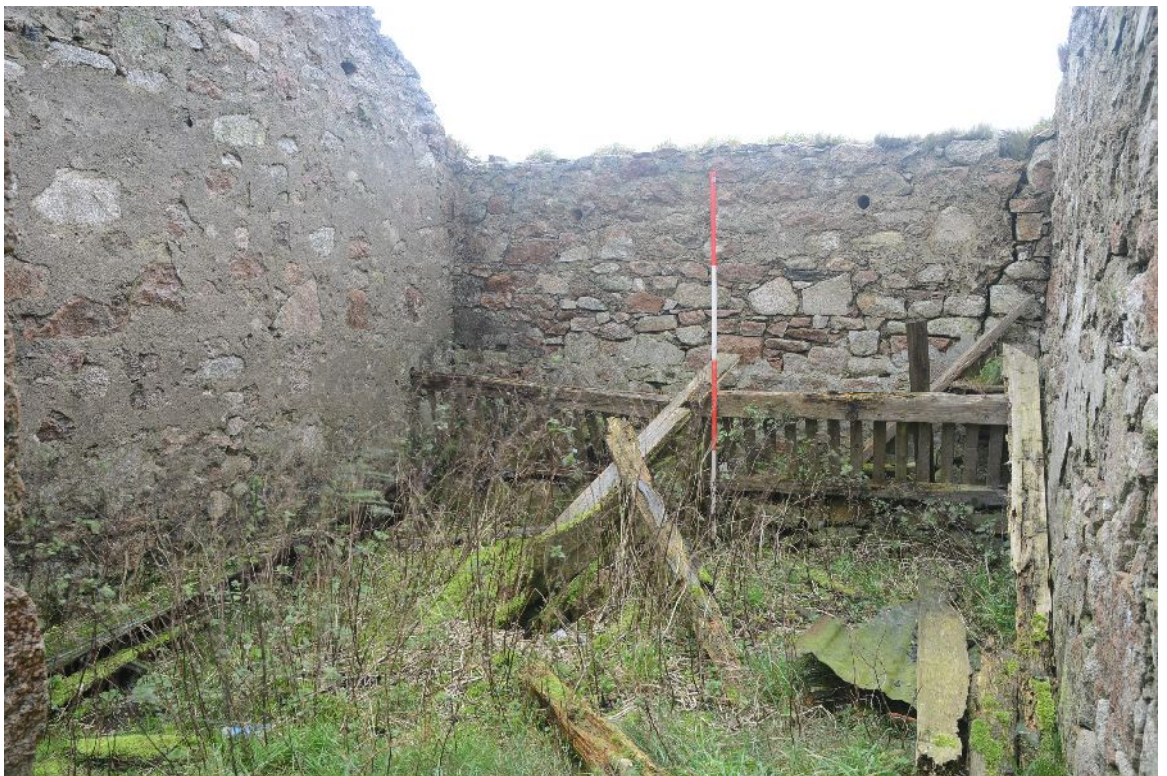
Illus 32 N Range looking N. Stable with ranging rod beside hay hake indicating the collapsed trevis.
