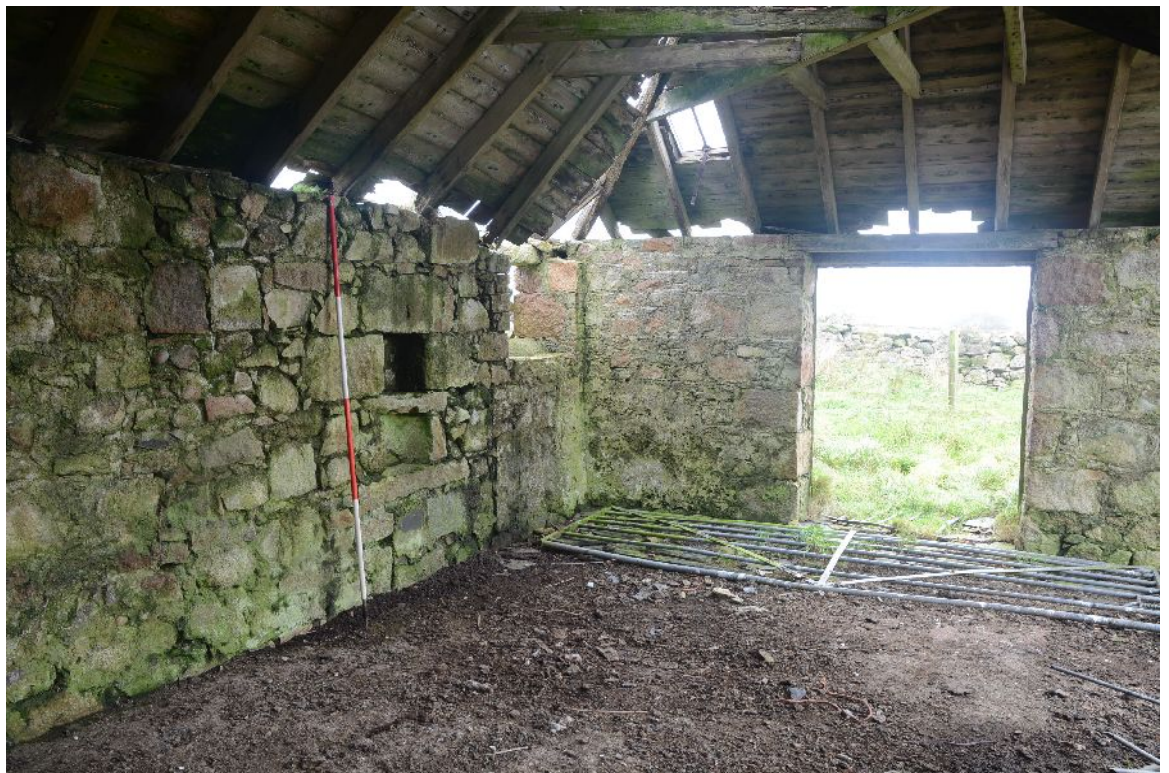
Illus 30 Interior of S Range, mill looking W. F1 & F2 beside ranging rod. Door D3 on RHS
