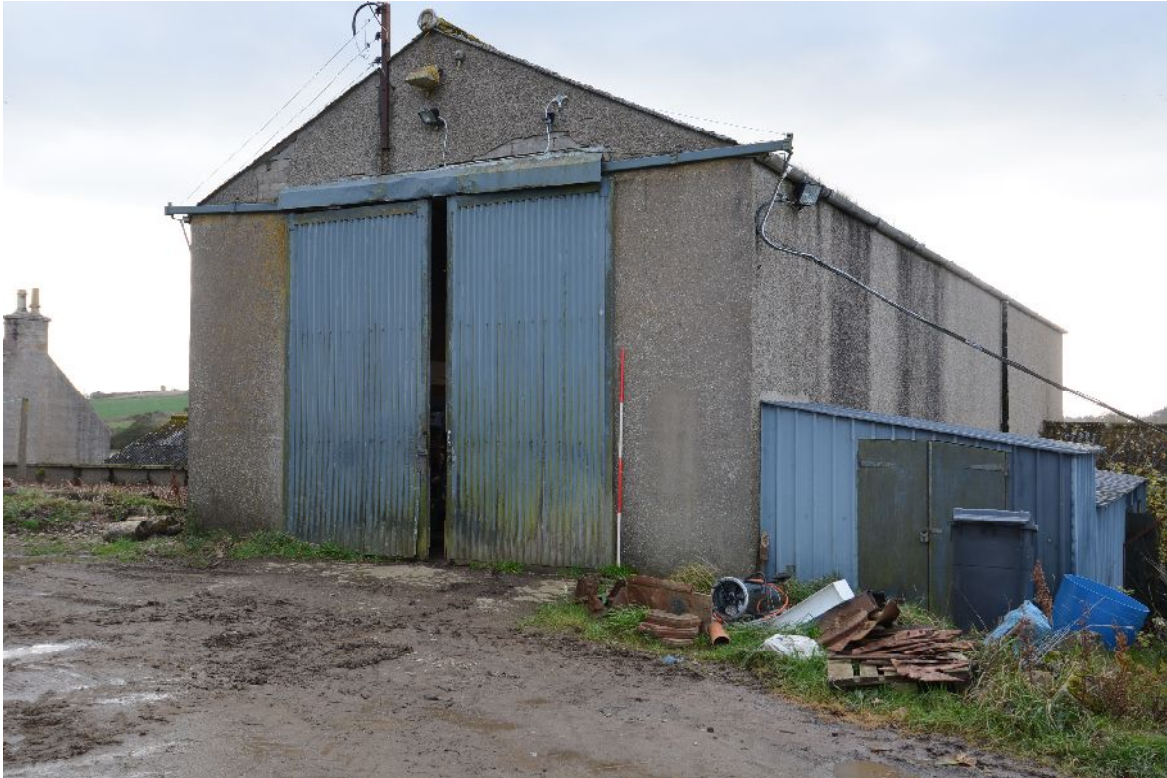
Illus 18 Building B central range with modern door D2 into heightened loft/first floor
