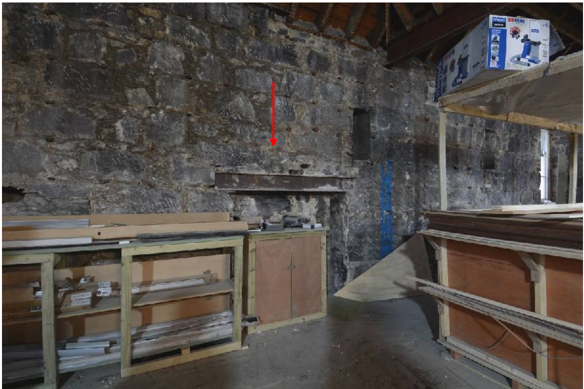
Illus 60 Arrow marks blocked fireplace (photo 9)
