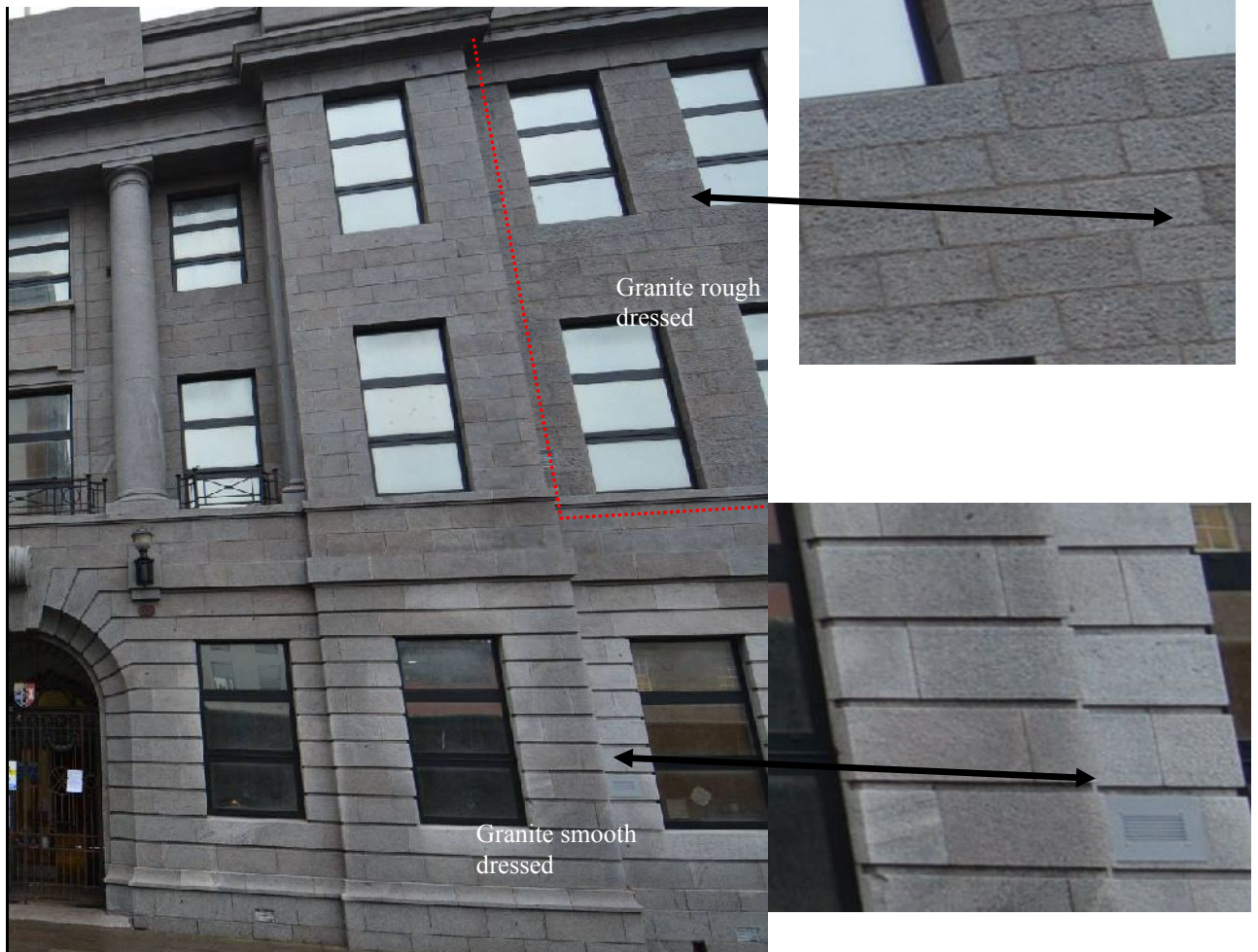
Illus 20 Detail of St Andrew Street facade showing difference in granite dressing
