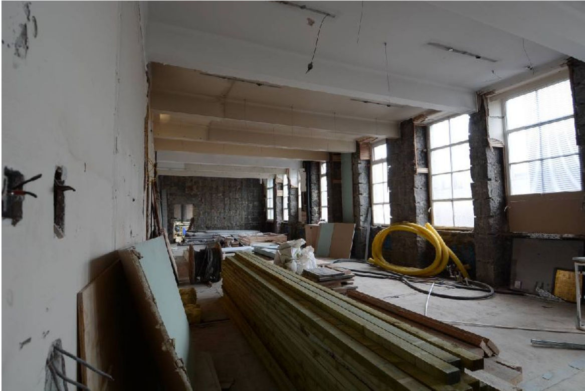
Illus 54 1 st floor. Looking SW along interior of John Street block. Windows to John Street. (photo 19)
