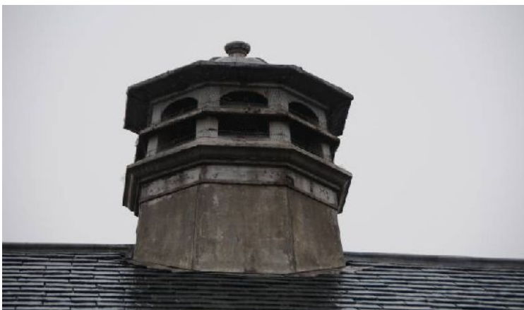
Illus 14 Ventilator (photo 18)
