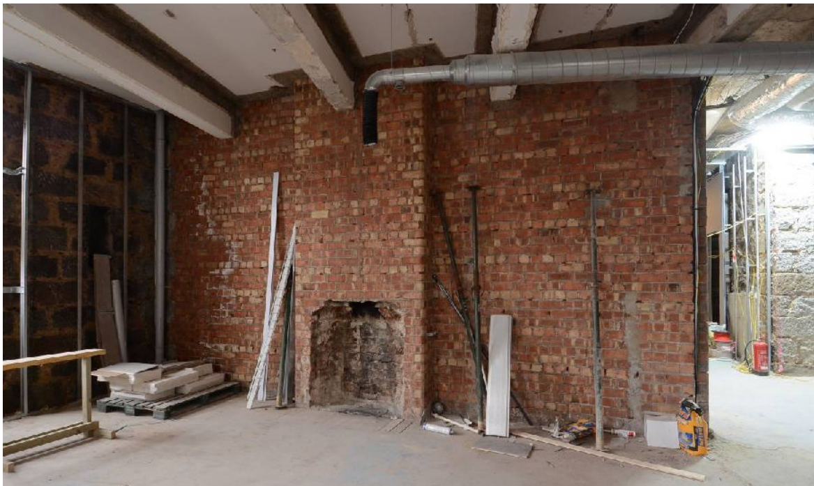
Illus 12 Original brickwork on ground floor. Charlotte Street/ St Andrew Street corner block, fireplace in SW wall (photo 31)
