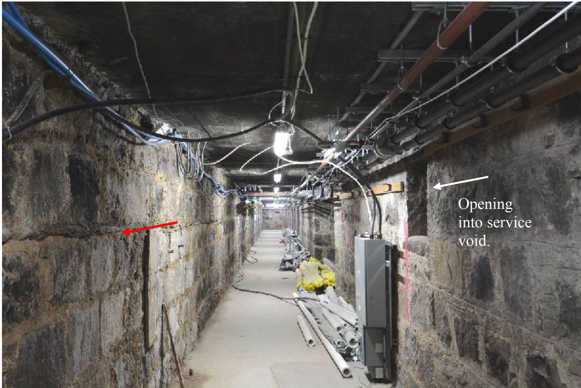
Illus 44 Basement passage parallel to North St Andrew Street. Red arrow indicates slate damp course. (photo 46)
