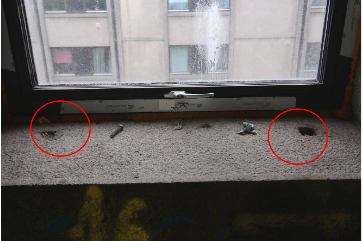
Illus 62 Scars (red circles) from the original railings now replaced by windows
