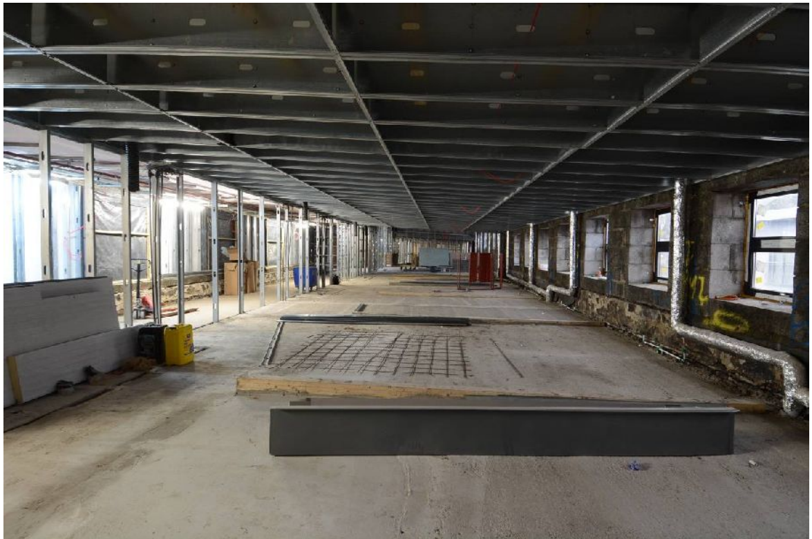
Illus 61 The Charlotte Street roof garden, now roofed. The windows on RHS replaced the original railings.
