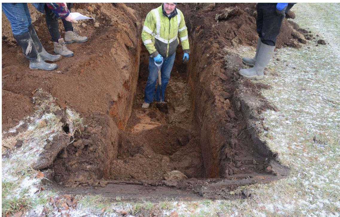
Illus 13 Service trench in test pit beside trench 3. Hand dug to a depth of c 1.4m from ground surface. Fill was stones and re-deposited topsoil.
