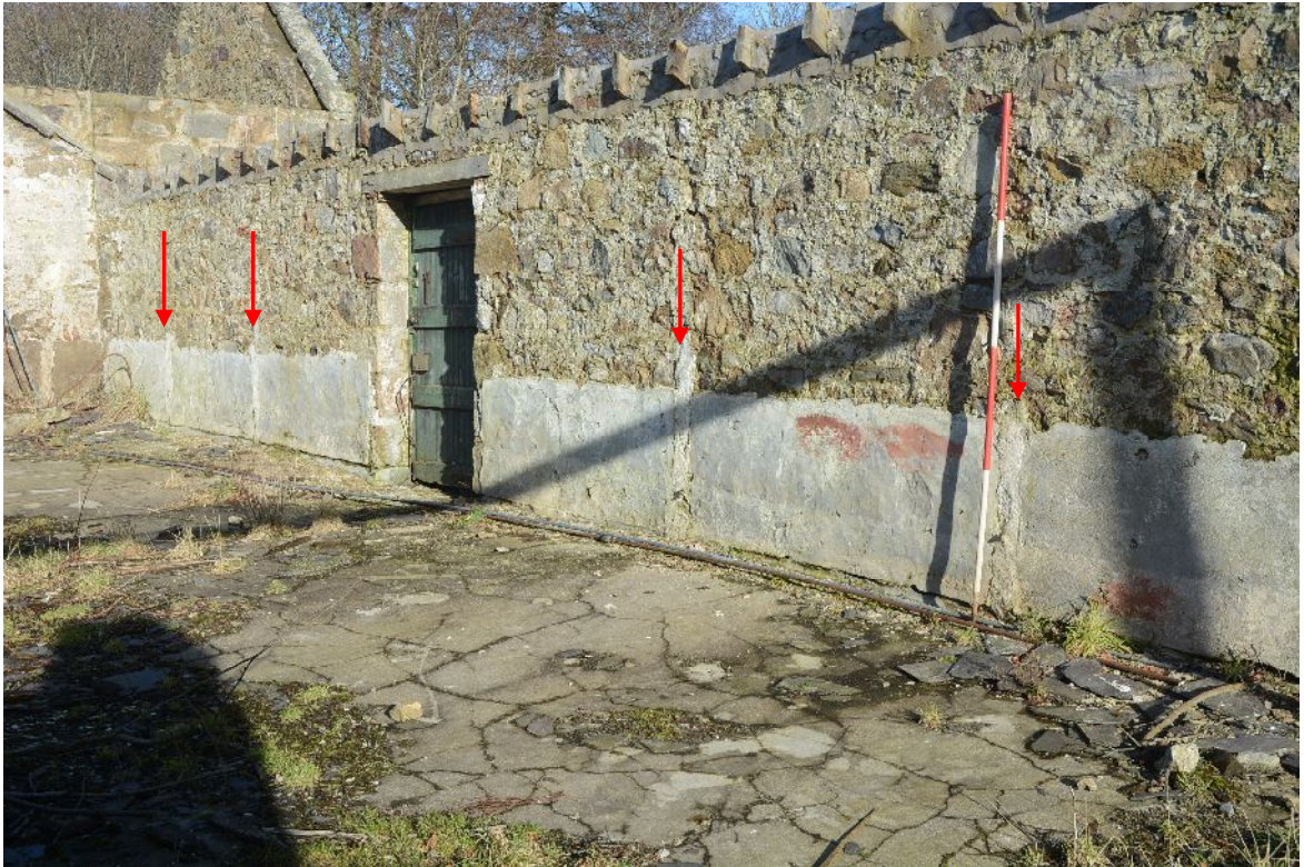
Illus 14 E Range. Inside of E wall. Arrows mark raggles of the divisions between the cow stalls.
