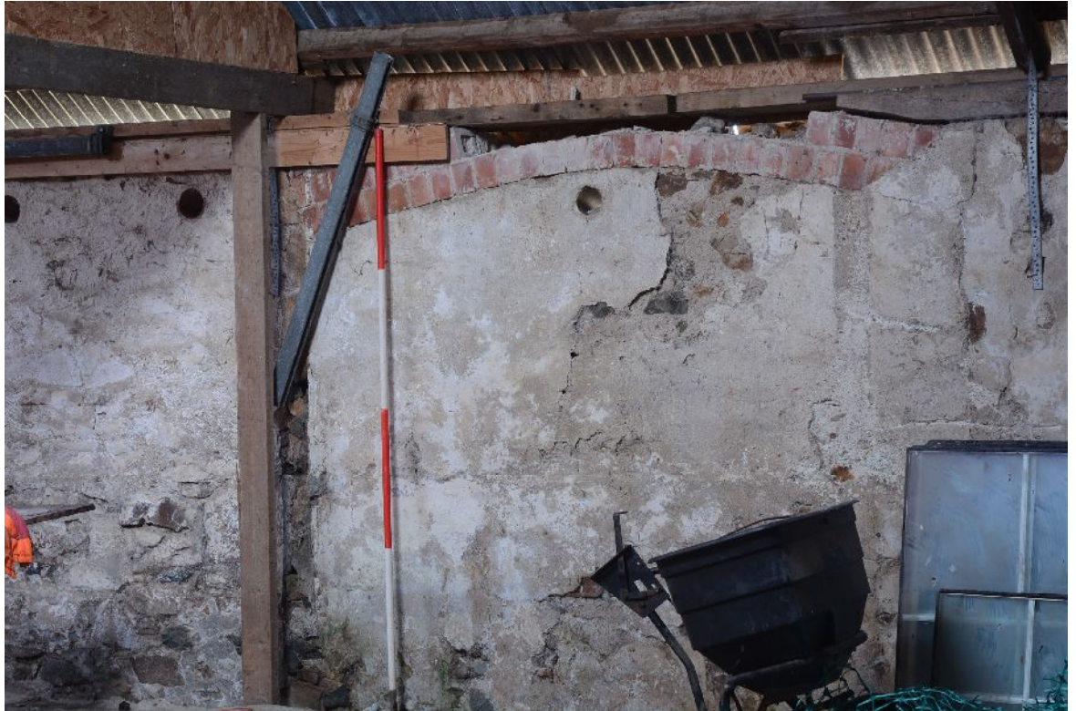
Illus 14 Interior of E Range, detail of inside of E wall, blocking of F3, plastering, ventilation pipe and scar of former partition (L of ranging rod).
