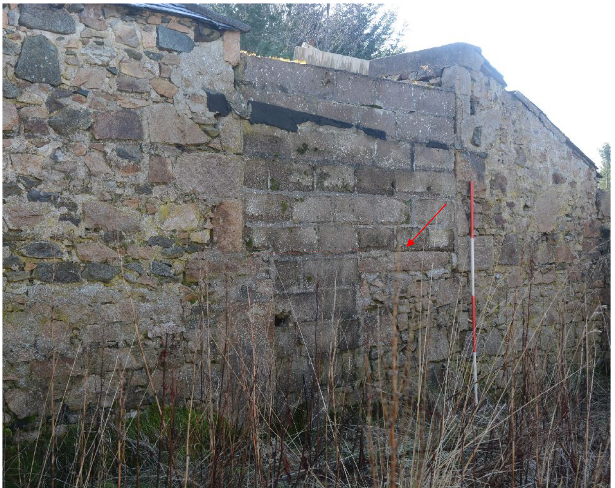
Illus 16 N wall of pig yard seen from inside dung court. Dotted line marks the blocked opening. The original , now displaced, lintel is marked with arrow.
