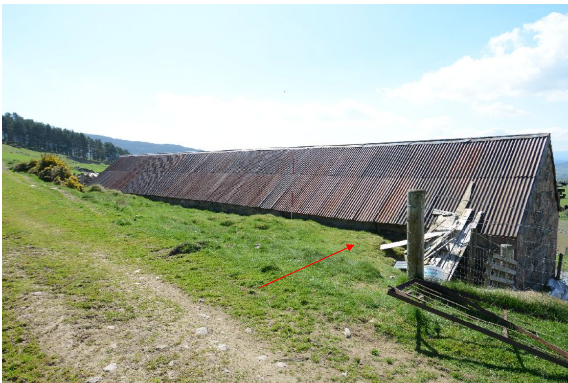
Illus 6 N wall of the steading, looking E. The approximate position of the horse mill shown on the 1899 OS map is indicated by a red arrow.
