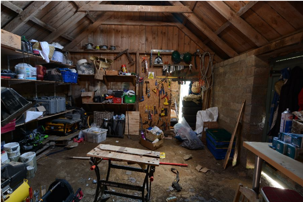
Illus 12 Interior of A, looking E to partition between A and B.
