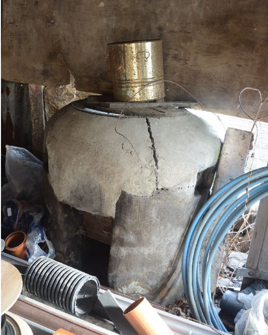
Illus 14 Wash-house boiler
