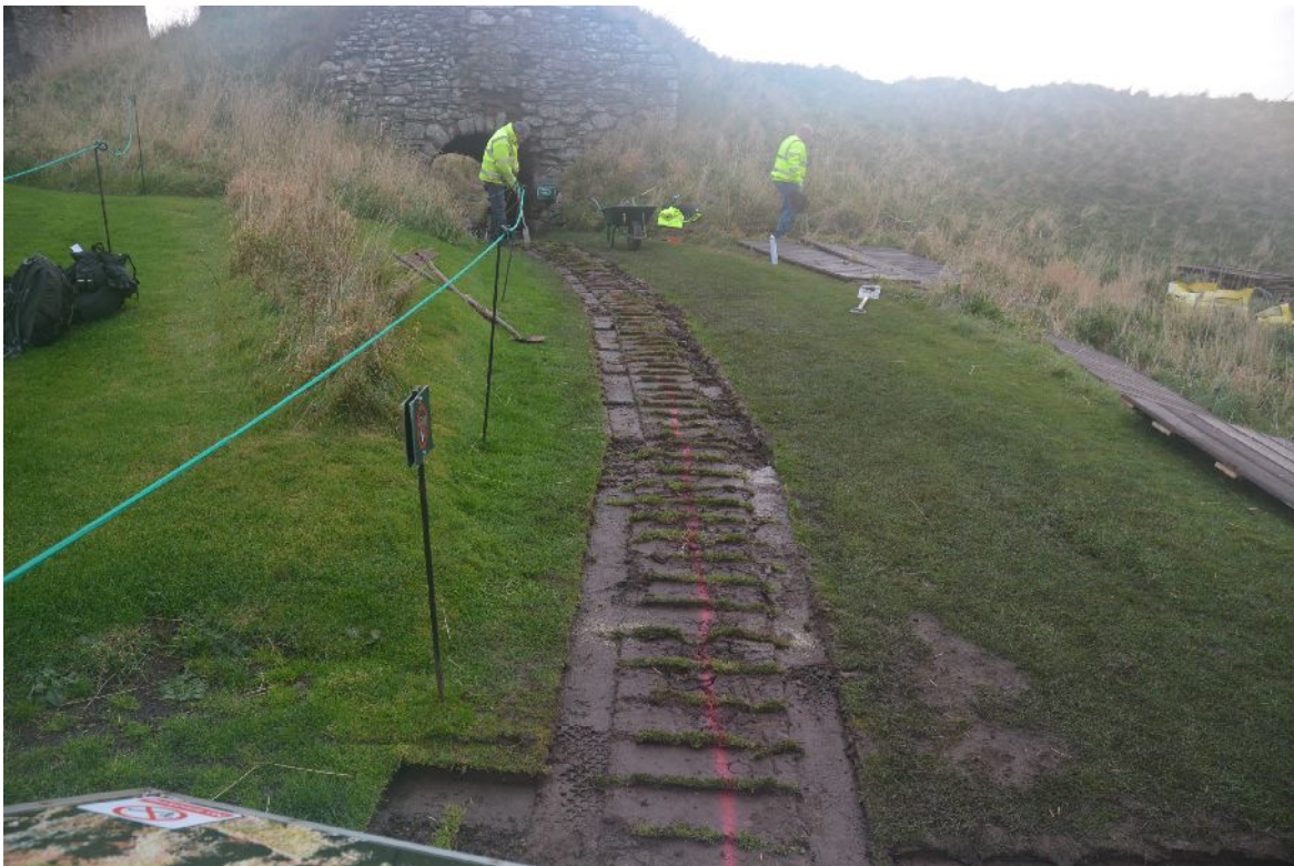
Illus 5 The walkway after removal of board walk, looking W to Pend entrance
