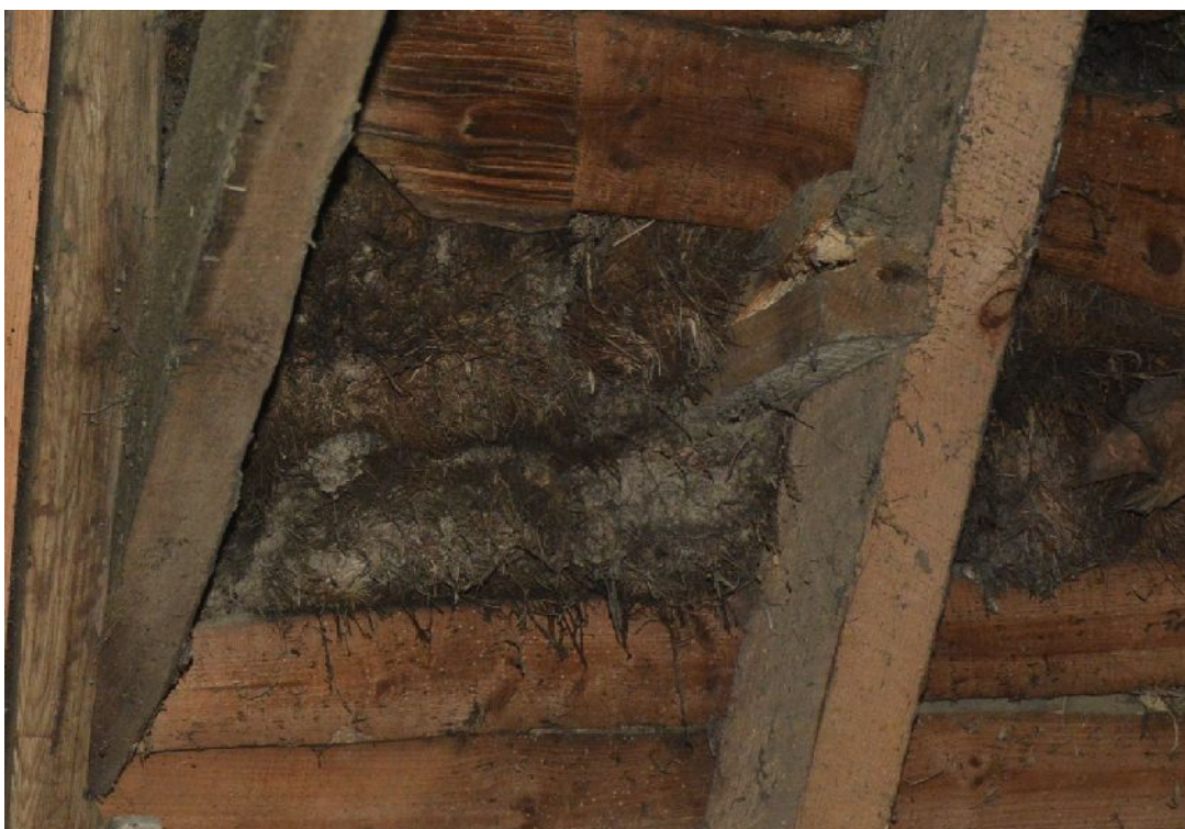
Illus 14 Detail of turves below corrugated iron
