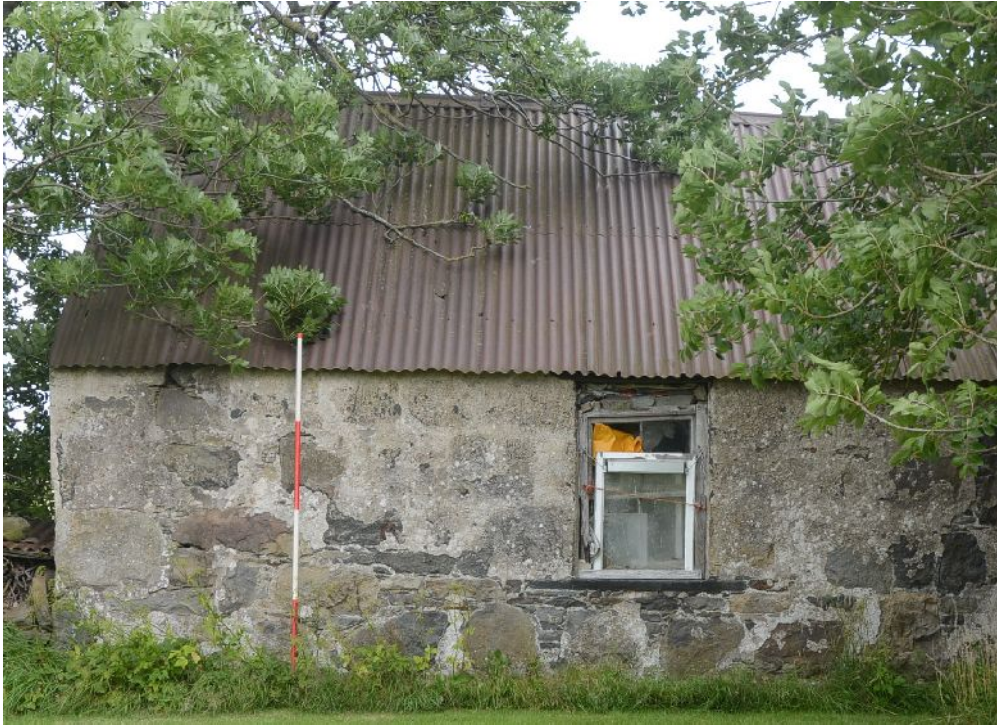
Illus 10 Detail of W end of S wall showing detail of stonework
