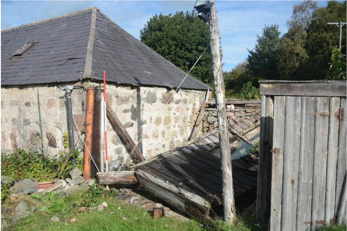
Illus 9 E gable and collapsed wooden structure
