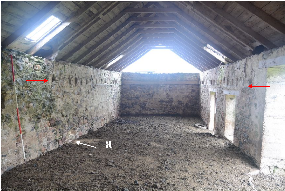
Illus 25 Building A (mill) looking N. Red arrows indicate the position of the loft. A= axle hole to wheel.
