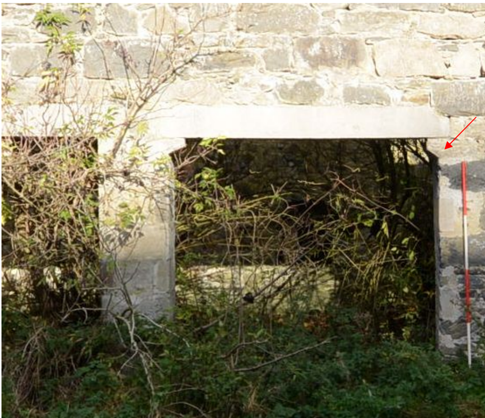
Illus 42 SW Elevation of mill. Detail of D6. Red arrow indicates line of arch replaced by concrete lintel
