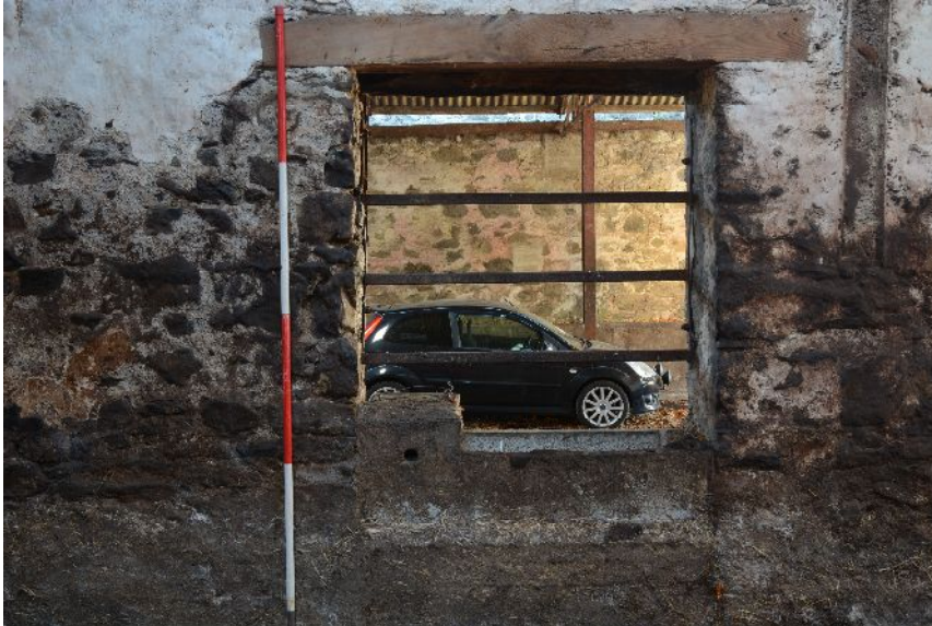
Illus 34 Door D7 from Area A showing partial blocking by water trough
