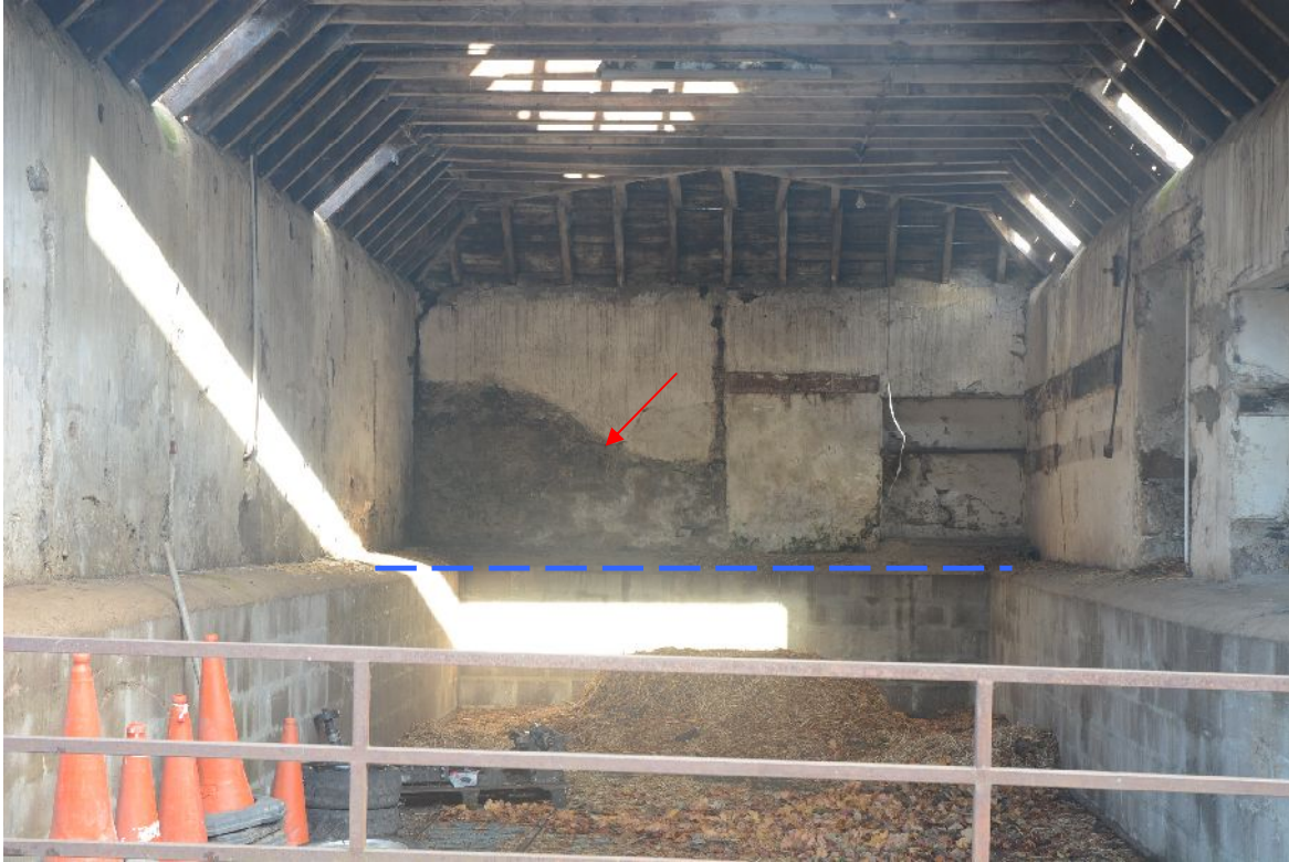
Illus 39 Looking NE into Building A. Red arrow indicates trevis mark. Blue line indicates original floor level
