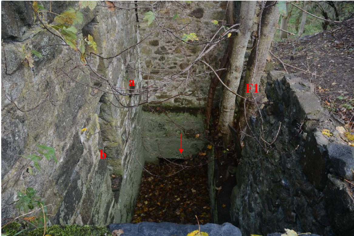
Illus 45 Looking NW along inside of wheel pit. Red arrow marks lade outflow. Openings a, b and F1 are marked
