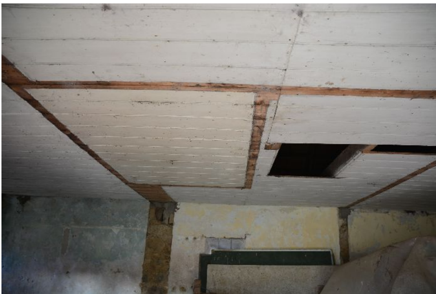
Illus 13 Interior. Looking from D1 at paint lines in ceiling which indicate former internal walls
