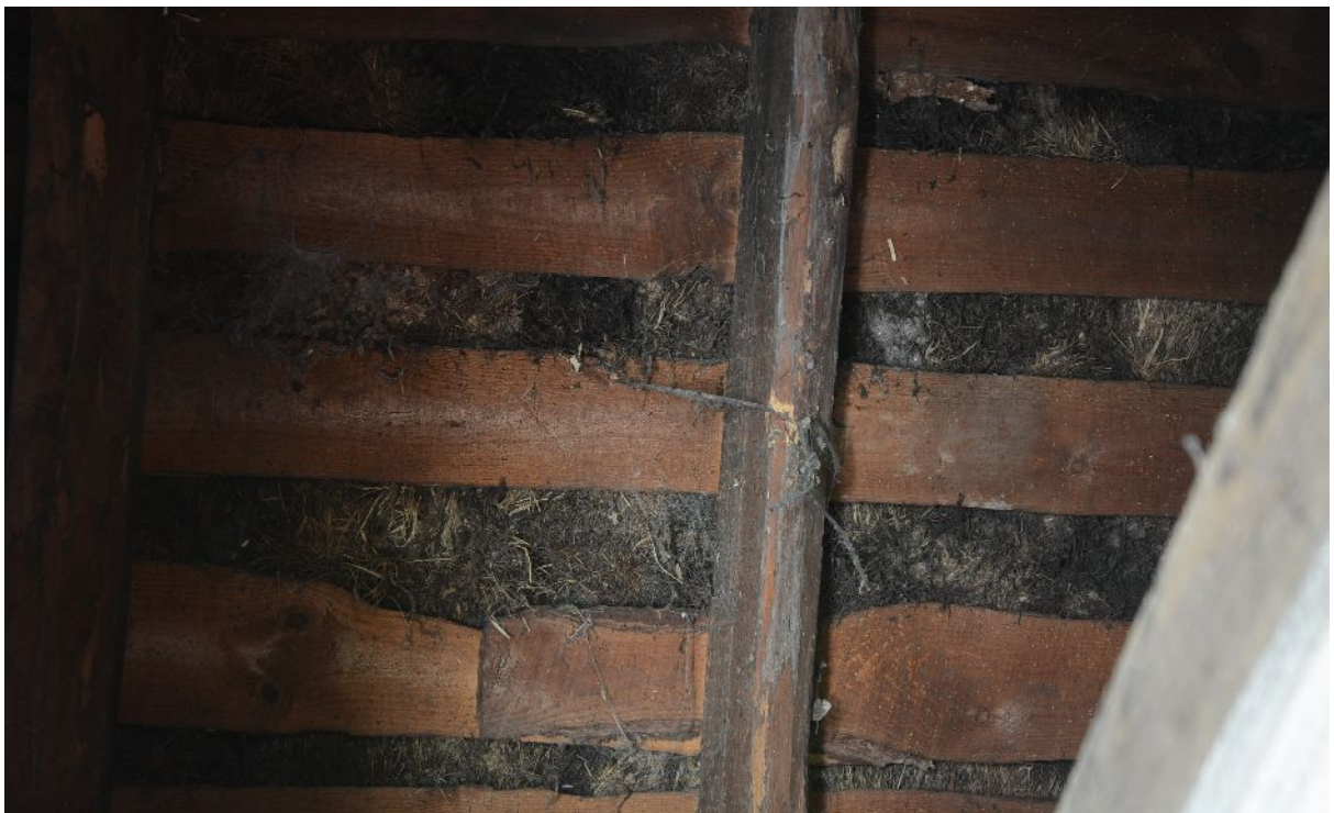
Illus 8 Turves visible below corrugated iron, seen through hatch in ceiling in lobby.
