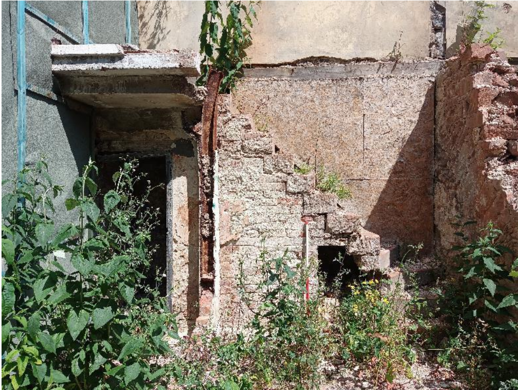
Plate 11: Staircase remains of the small cottage at north-west end of site
