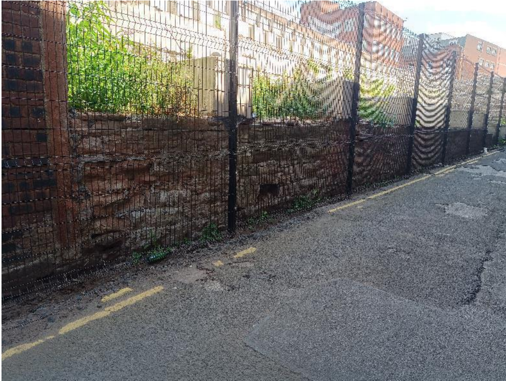
Plate 14: Remnants of foundation or boundary wall, with lower street level
