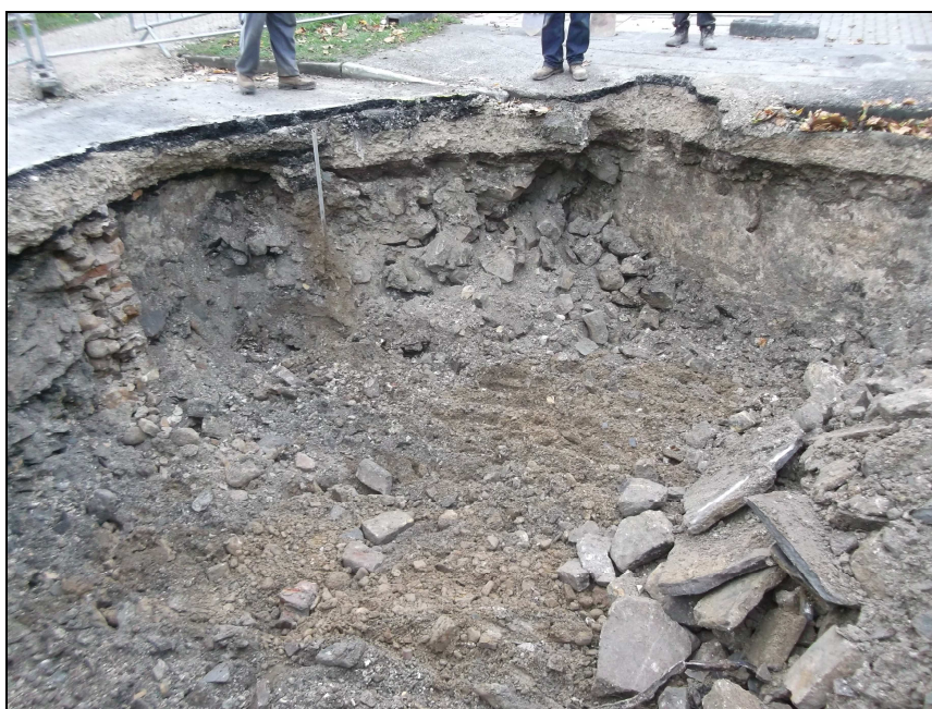
Plate 6: Photograph of brick walls [010] in rubble (009) beneath road surface of Lune Street
