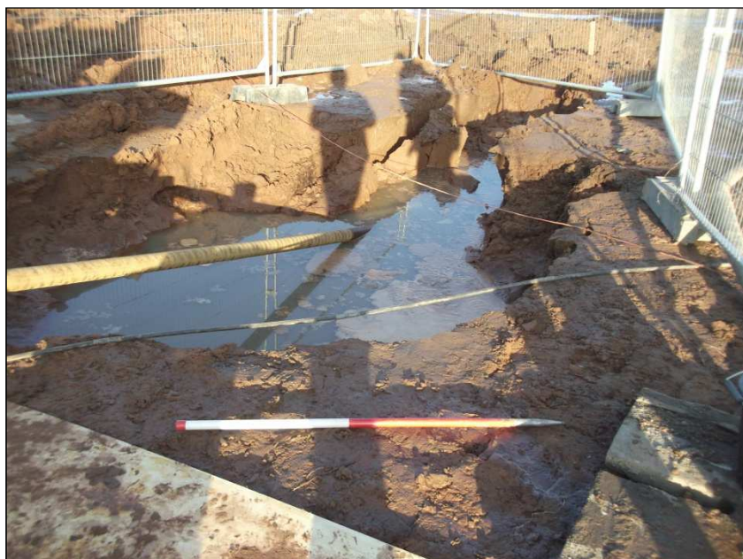
Plate 12: Area 3, horizontal boring trench on the western side of the M6 motorway (facing north-east)
