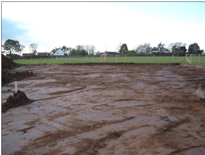
Plate 1: Area 1, topsoil stripped area at the western end of the pipeline (facing west)
