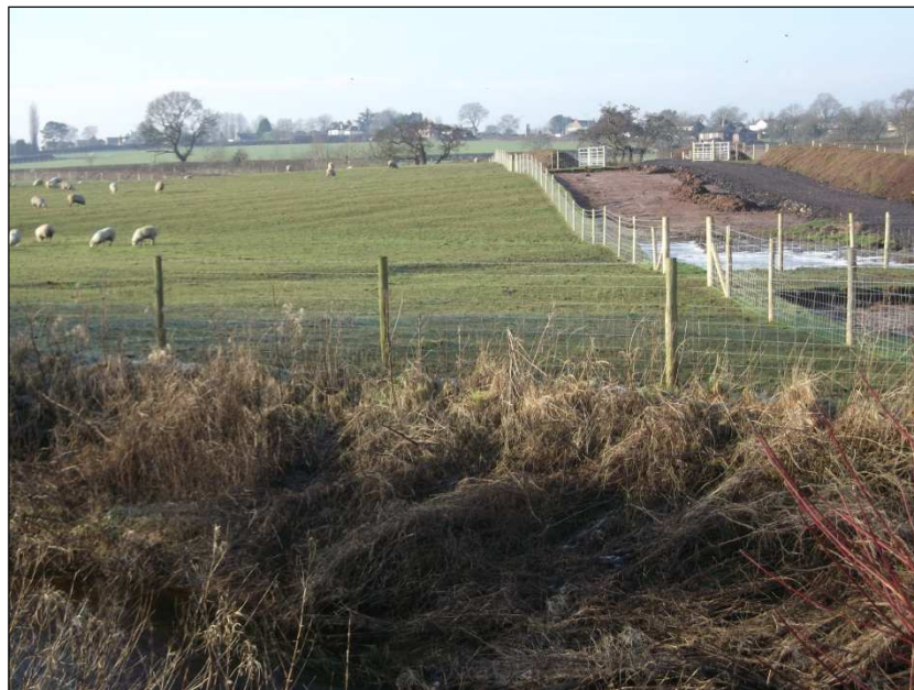
Plate 2: Area 2, pipeline easement cutting narrow ridge and furrow at the northern end of the field (facing west)
