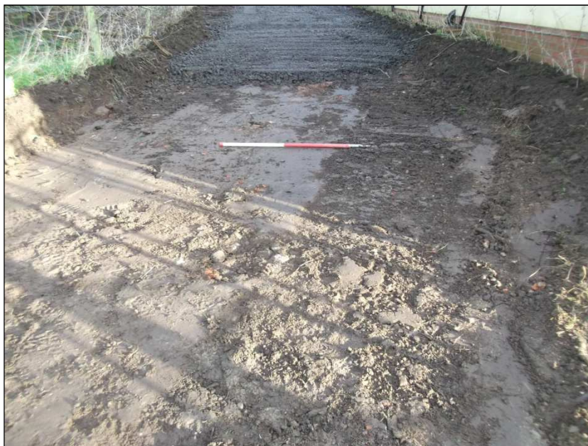
Plate 8: Area 12, modern rubble observed during access road excavation, adjacent to Low Crosby Village (facing north)
