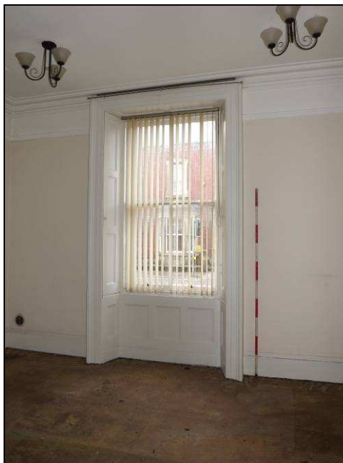
Plate 26: Detail of window in west wall of Room G1, ground floor (Scale = 2m)
