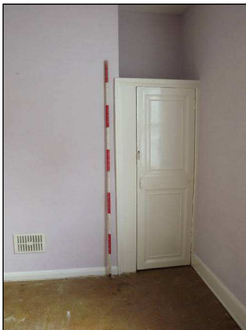
Plate 41: Detail of cupboard, Room F4, first floor of rear wing (Scale = 2m)
