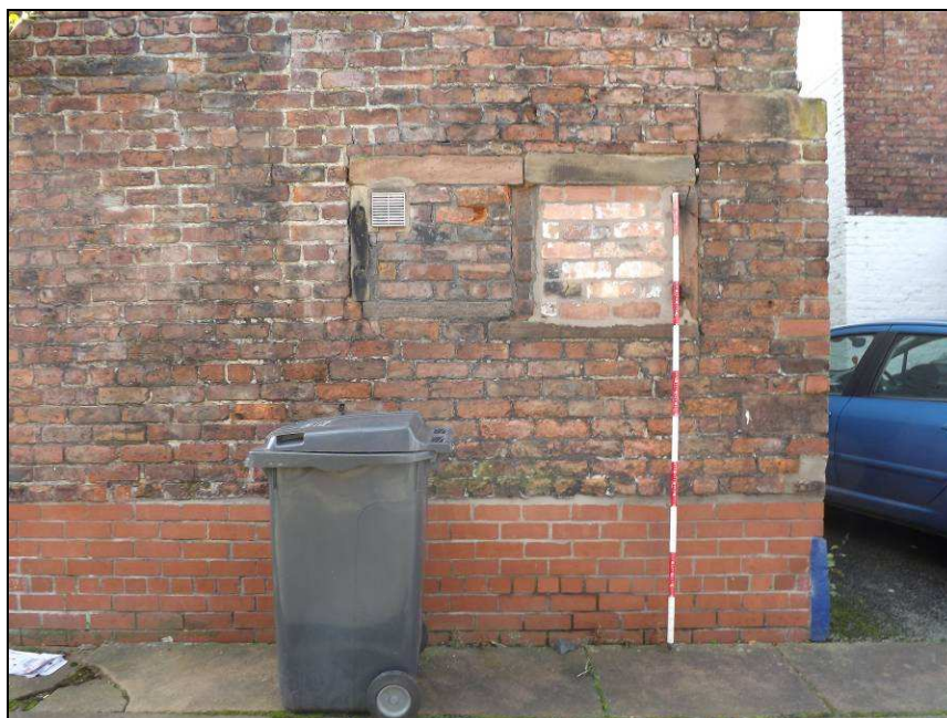
Plate 14: Detail of blocked up 'coal holes', rear of 7 Spencer Street (Scale = 2m)
