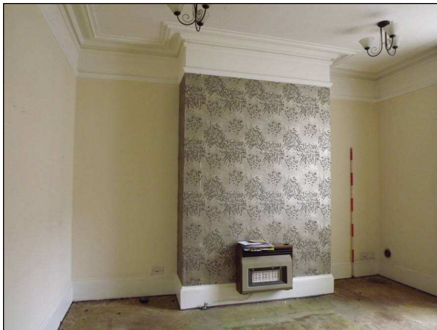
Plate 28: South wall of Room G1 showing coving, picture rail and chimney breast (Scale = 2m)
