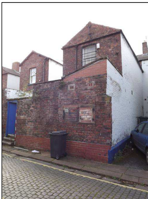
Plate 13: Rear of 7 Spencer Street showing the varying brickwork of periods of reconstruction and alteration
