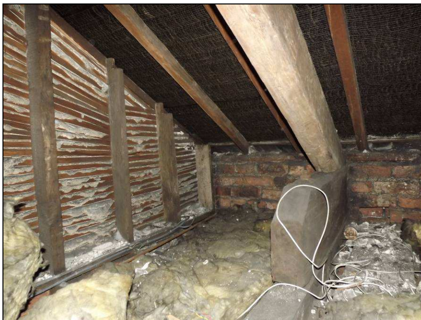
Plate 59: Detail of roof structure and lathe and plaster wall as seen in the eastern void of the roof
