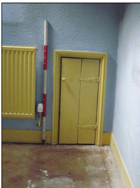
Plate 57: Detail of access door into roof void, west wall of Room S1 (Scale = 1m)
