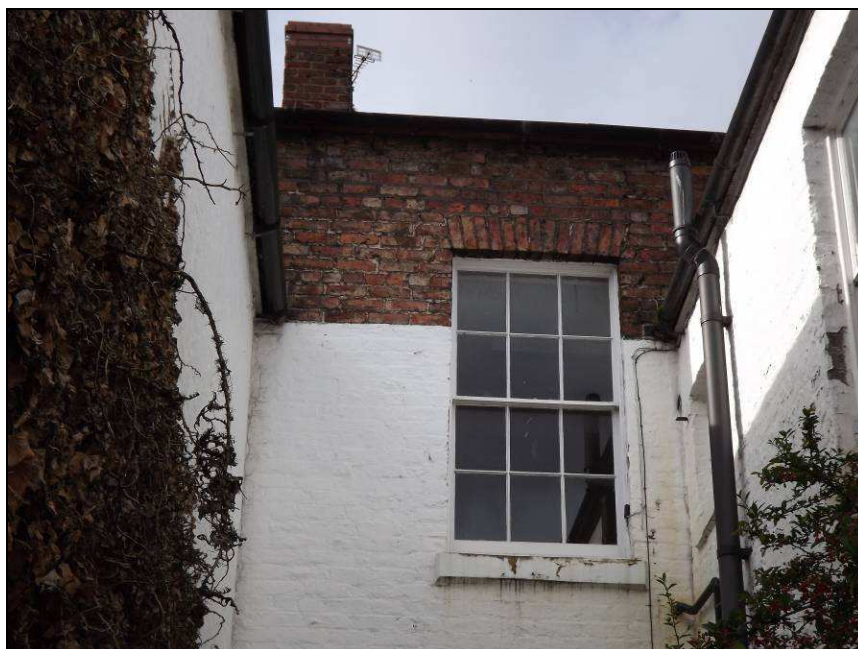
Plate 16: Detail of first floor window (lights Room F1), east elevation as seen from yard to rear of 7 Spencer Street
