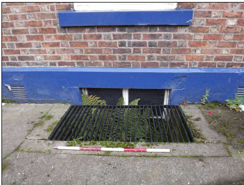
Plate 11: Detail of window which lights the basement of No. 5 Spencer Street (Scale = 1m)
