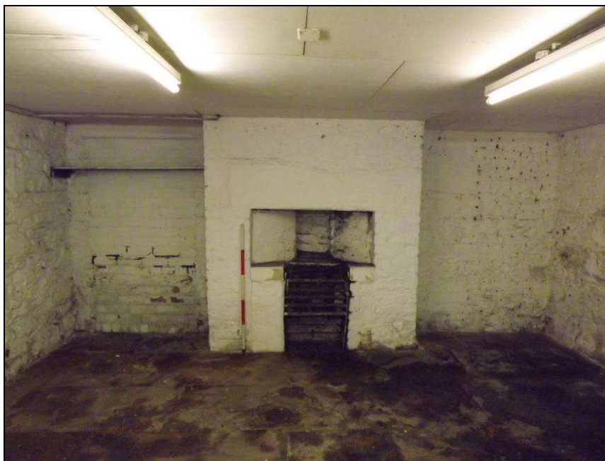
Plate 65: South wall of Room B1 in basement, showing fireplace with blocked door to left hand side (Scale = 1m)
