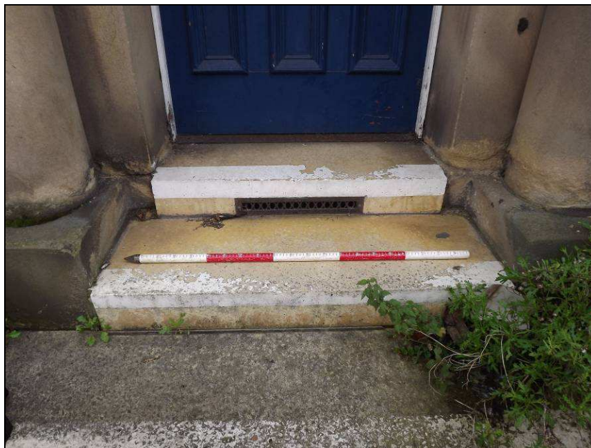
Plate 8: Detail of stone steps to main doorway and ventilation grill for the basement (Scale = 1m)
