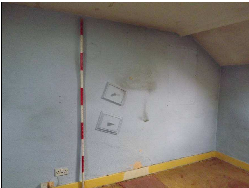
Plate 56: South wall of Room S1 showing metal plates for possibly cleaning chimney (Scale = 2m)
