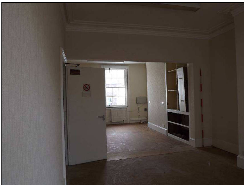
Plate 44: View looking east towards Room F1 from Room F2 showing area of removed wall
