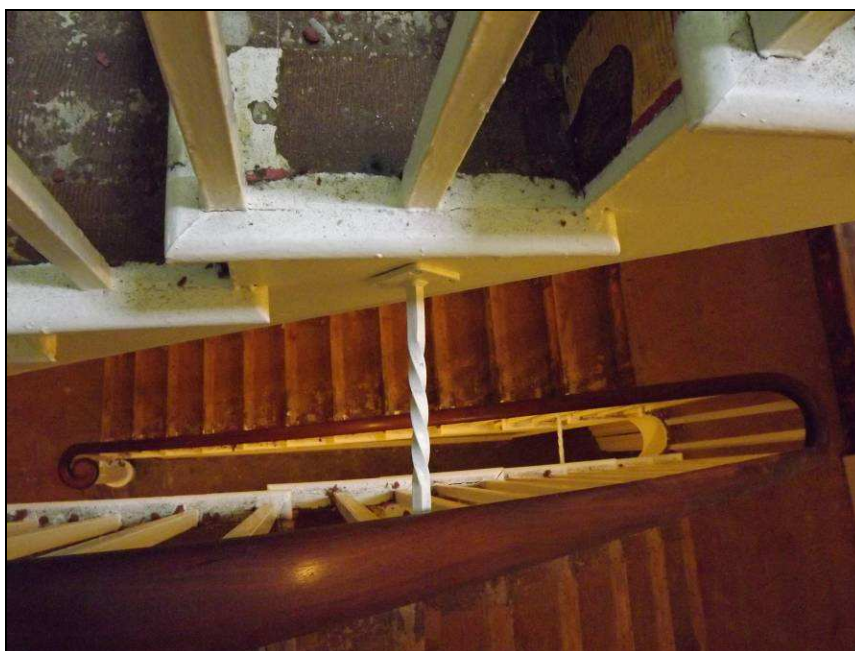
Plate 43: Detail of iron bars between the dog-leg staircase as seen from first floor
