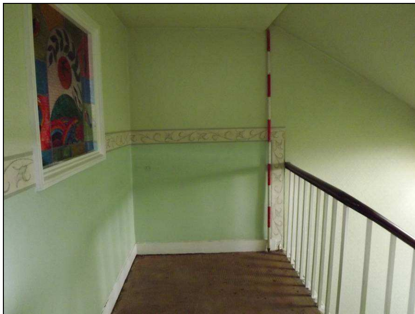
Plate 54: View looking north showing the location of the second floor within the roof space (Scale = 2m)
