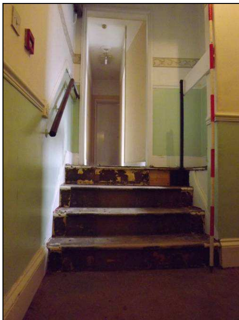
Plate 40: View looking east showing the stairs to the first floor of the rear wing
