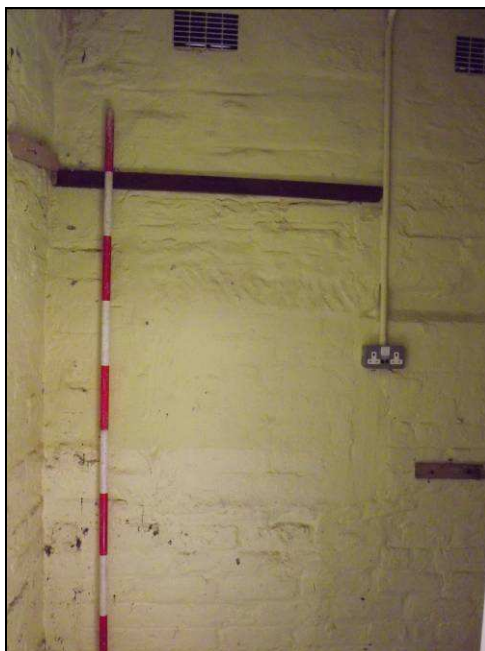
Plate 39: Detail of blocked 'coal hole' as seen from the store to the east of Room G4, ground floor
