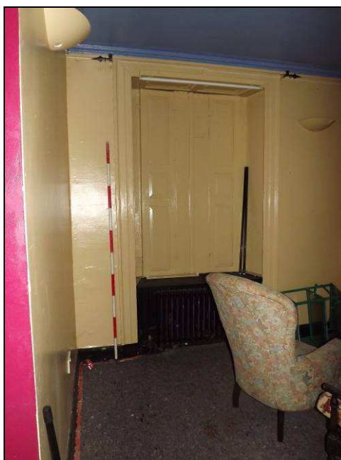
Plate 39: One of the two windows in the north wall of Room 3 (Scale = 2m)
