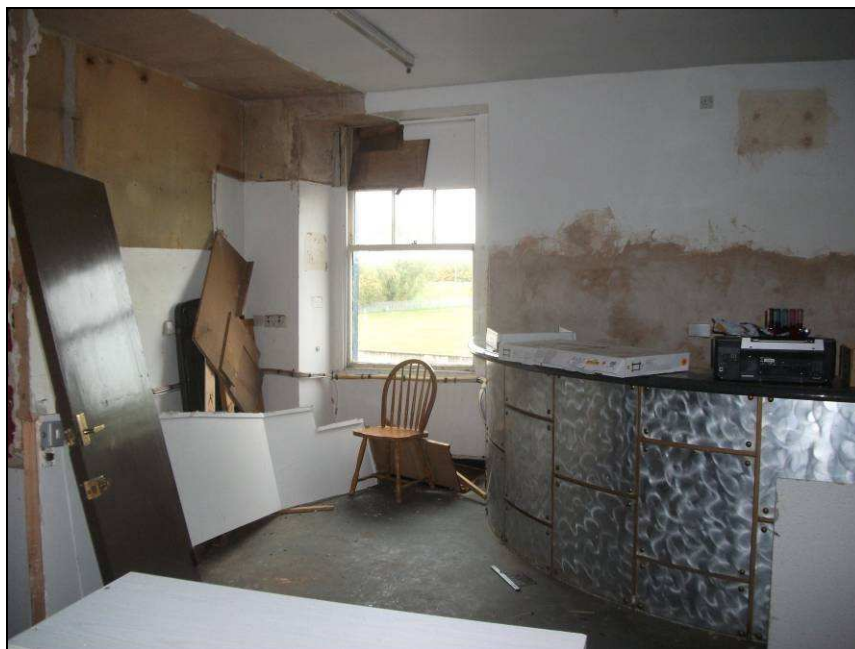
Plate 46: Western window in Room 4 showing lower section with missing glazing bars
