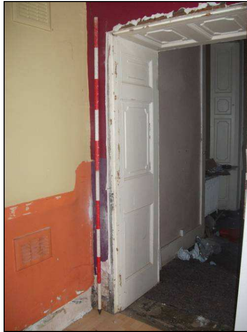
Plate 28: Detail of original door case between Rooms 1 and 2 (as seen from Room 2), Ladies' Walk Level
