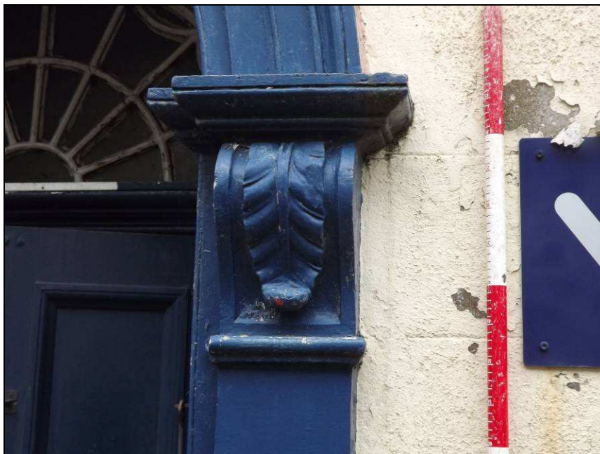
Plate 11: Detail of one of the consoles of the original doorway, south elevation
