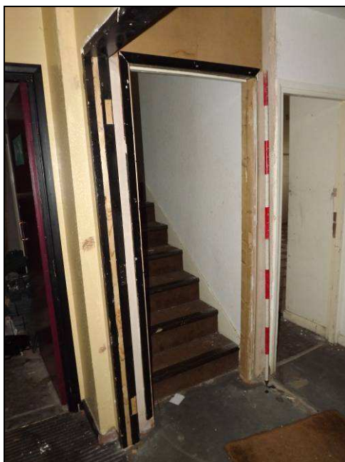
Plate 49: Detail of inserted staircase, south side of Rooms 5 and 5 on Ladies' Walk Level
