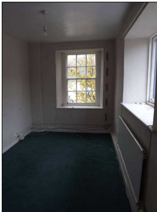
Plate 56: View looking east showing an historical window in the east gable, first floor level
