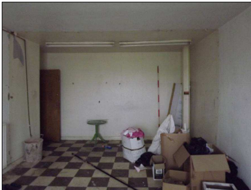
Plate 51: View looking south showing the interior of Room 6 with steel beam in south-west corner
