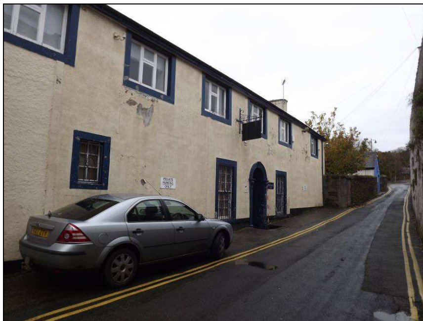
Plate 14: South elevation showing possible original small ground floor window to left of photograph, with vertical projecting to its west side
