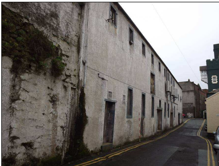
Plate 65: View looking west down Ladies' Walk showing the former brewery building on the south side of the street
