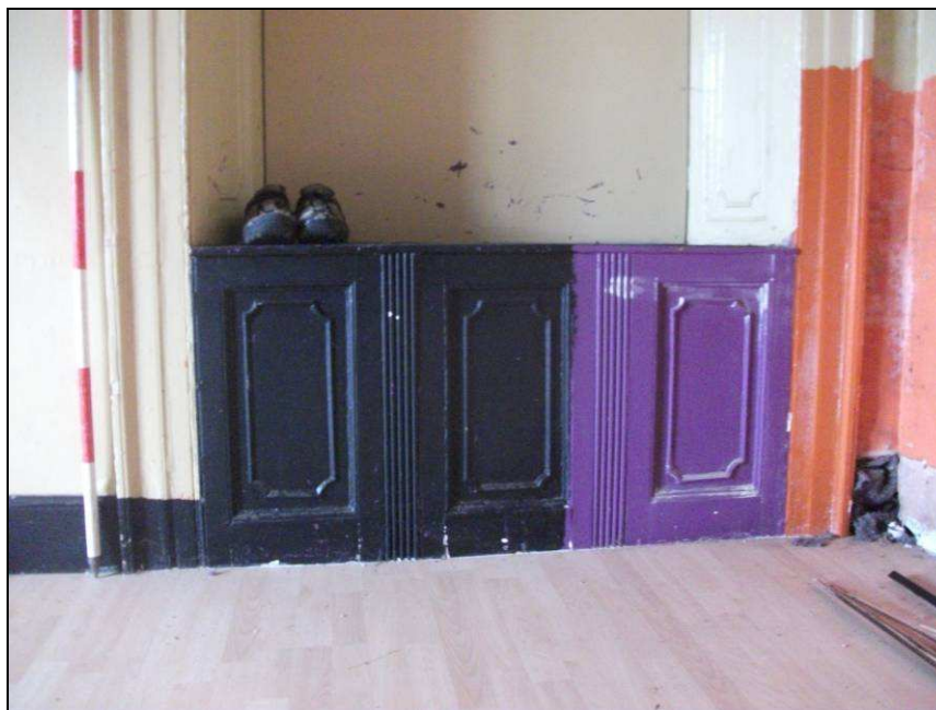
Plate 34: Reused panelling for a sill for a window in the east wall of Room 2
