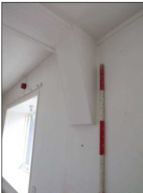
Plate 54: Detail of one of the boxed-in ends of a roof truss, first floor level
