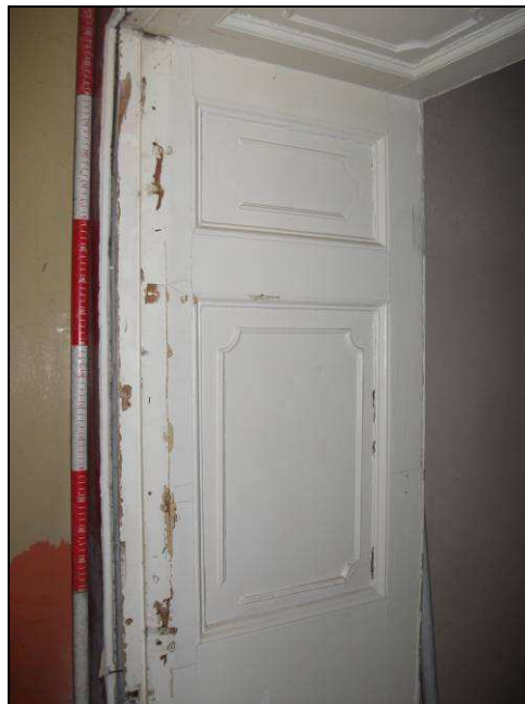
Plate 29: Detail of the panelling of the door case between Rooms 1 and 2, Ladies' Walk Level
