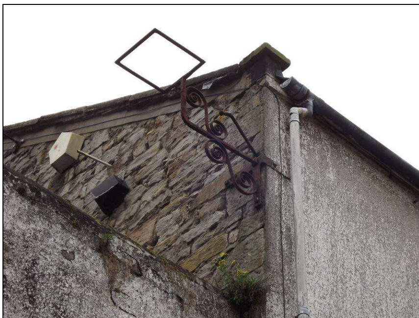
Plate 66: Detail of kneeler on east gable of former brewery building, south side of Ladies' Walk
