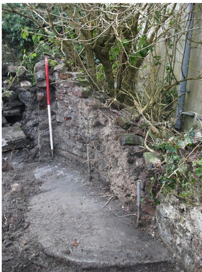
Plate 14: View of windmill {501} looking southwest, showing height of structure and blocked doorway
