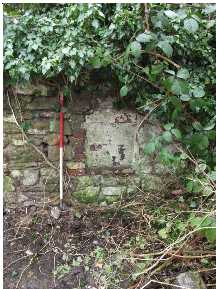
Plate 20: Close up of blocked window from site in {506}
