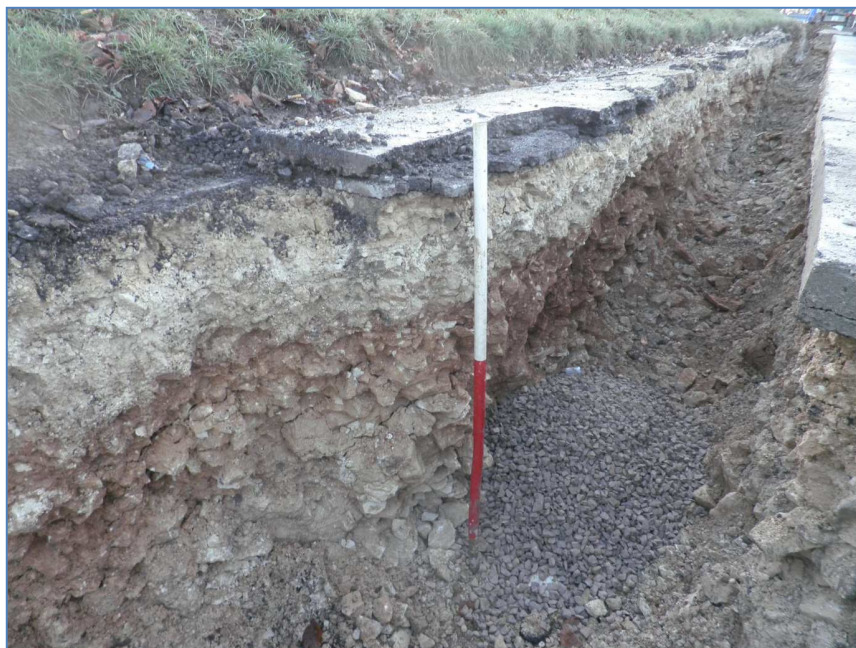
Plate 3: Looking south down open cut replacement trench, showing tarmac (101), made ground (102), and truncated limestone bedrock (103)
