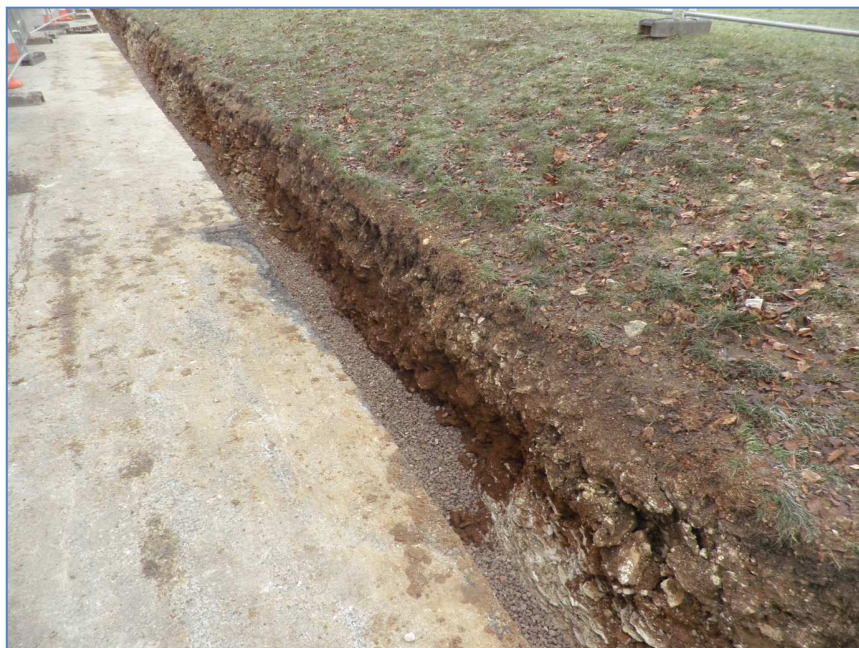
Plate 6: Looking northeast at the fully truncated profile of ditch [9], with fresh aggregate in base of replacement trench
