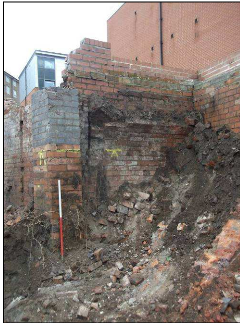
Plate 14: Shot of kink in west wall {1021} with arching brickwork
