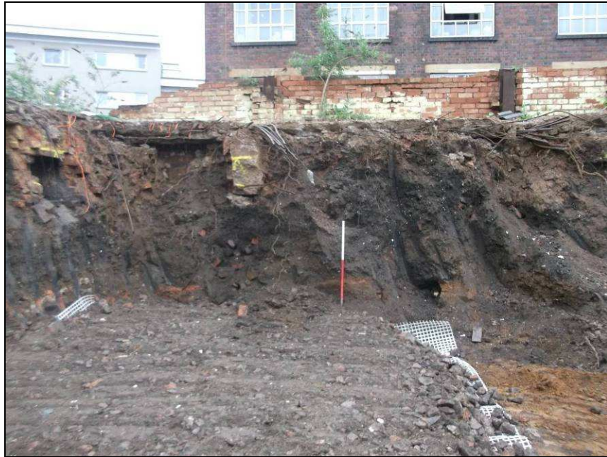
Plate 9: North facing shot taken in the north-west corner showing north wall with reinforced girders
