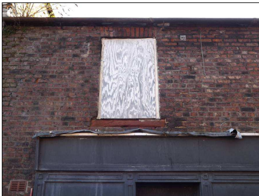
Plate 20: Detail of first floor window, north-west elevation of No. 3 South Henry Street
