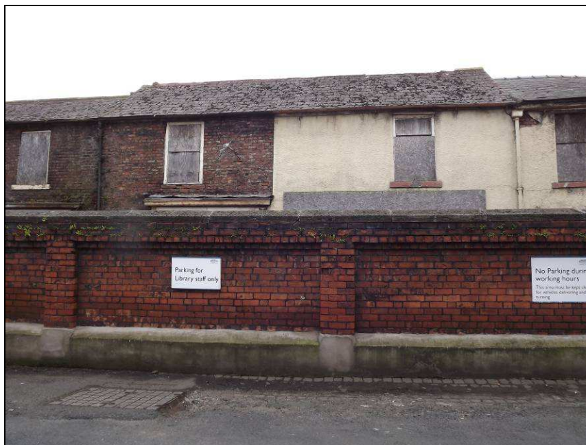
Plate 25: North-west elevation of No.1 South Henry Street as seen from the Library Services Car Park
