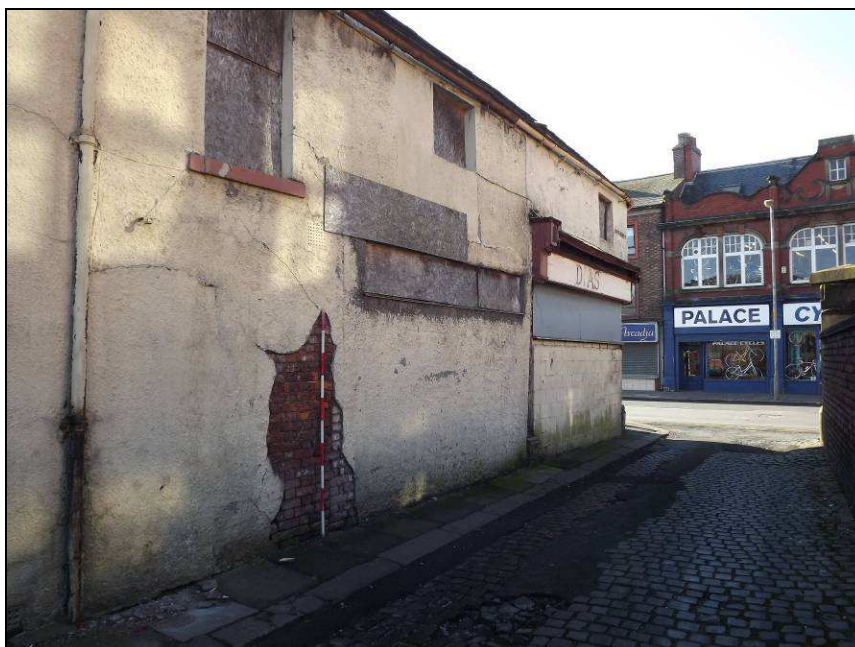
Plate 34: South Henry Street side of No. 149 Botchergate showing exposed brickwork (Scale = 2m)
