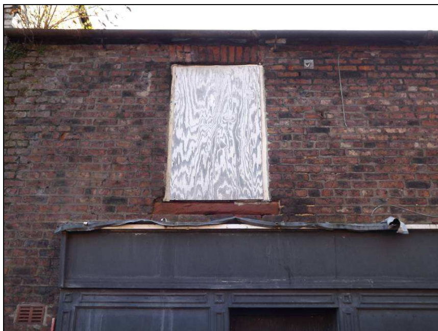
Plate 20: Detail of first floor window, north-west elevation of No. 3 South Henry Street
