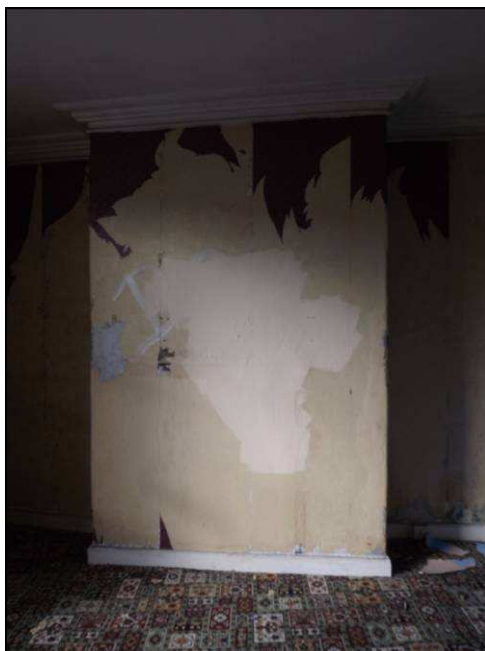
Plate 65: Detail of one of the chimney breasts, first floor of No. 155 Botchergate
