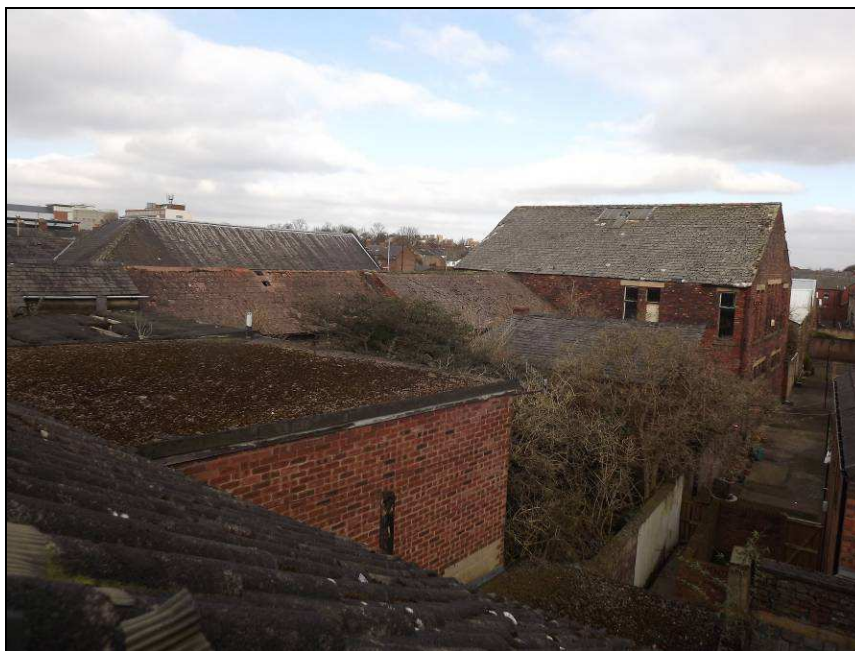
Plate 59: Detail of flat-roofed extension to the rear of No. 153 Botchergate (left of photograph) as seen from the roof space of No. 157
