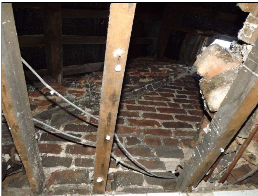
Plate 23: Diagonal line of an earlier gabled roof visible at the west end of No.2 South Henry Street, first floor level
