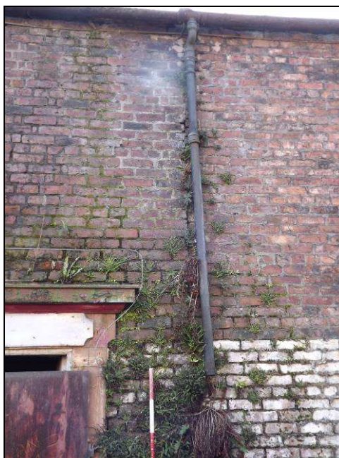
Plate 26: Vertical construction break between No's 1 and 2 South Henry Street
