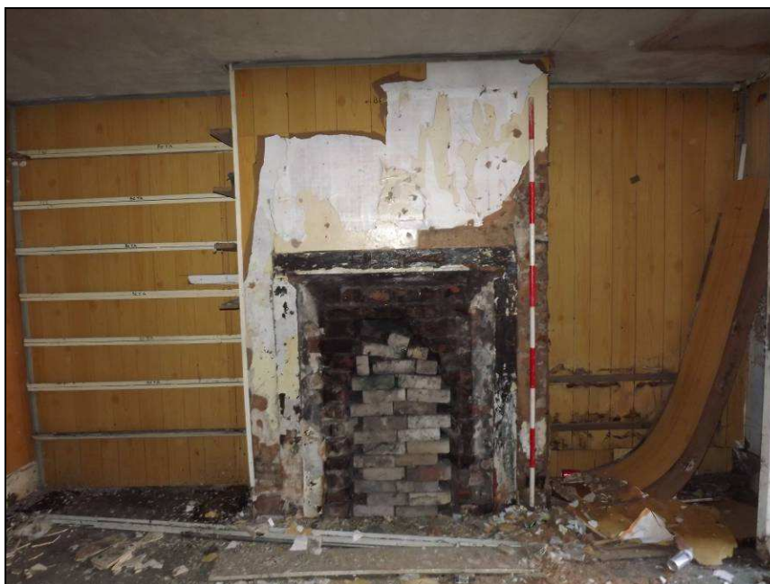
Plate 22: Detail of fireplace, ground floor of No. 2 South Henry Street (Scale = 2m)
