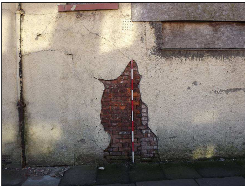
Plate 35: Vertical break in brickwork, South Henry Street side of 149 Botchergate
