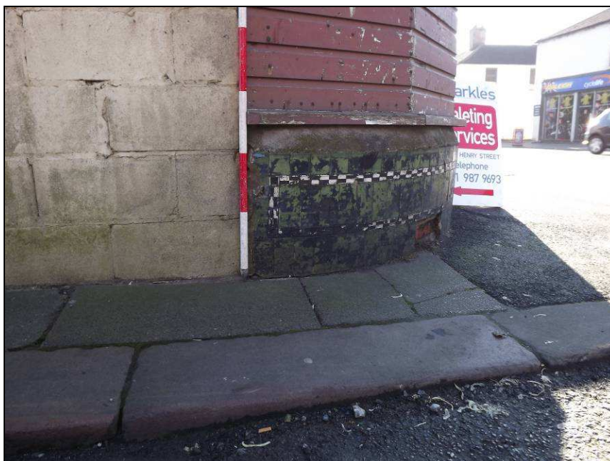
Plate 38: Detail of tiling on the corner of South Henry Street and Botchergate
