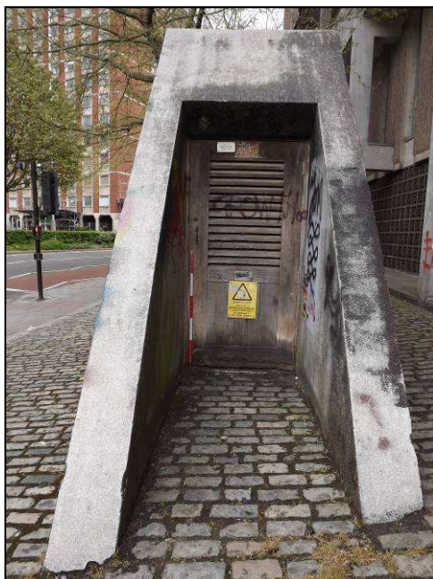
Plate 15: View looking north-east showing the access door to the electricity substation, north-west side of Magistrates Court
