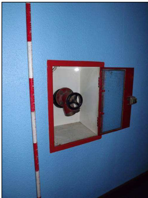
Plate 54: Fire hydrant, Fourth Floor
