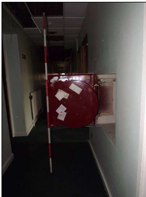
Plate 52: Detail of fire hose reel, Third Floor
