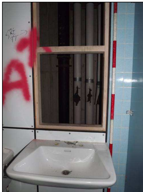
Plate 50: Detail of pipework hidden within ladies toilets, Third Floor
