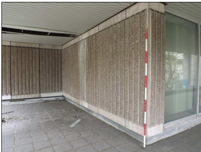
Plate 8: Detail of 'cladding' effect created by grooves cut into the concrete panels, and pebble-dashing, as seen at second floor level, south-west elevation
