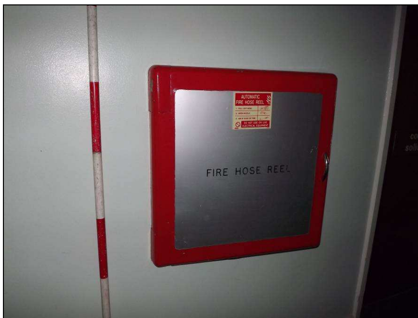
Plate 51: Detail of fire hose reel storage, Third Floor
