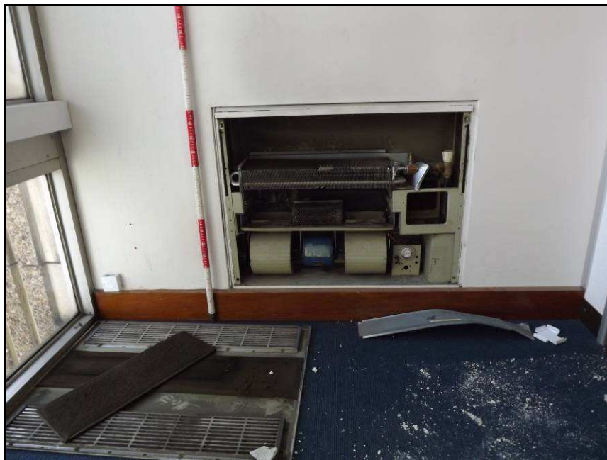
Plate 58: Detail of electric heater, Fourth Floor
