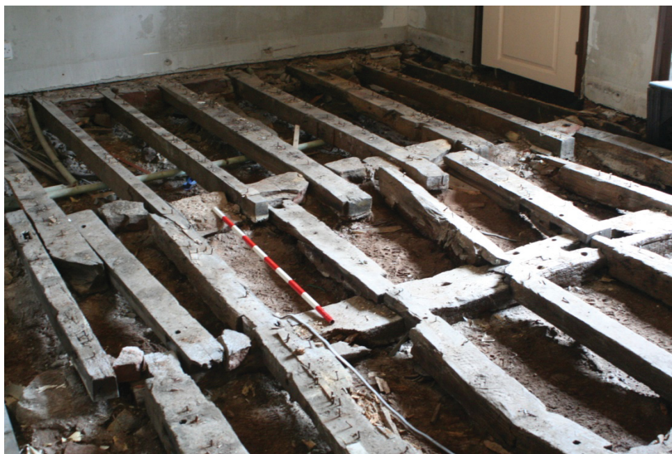
Plate 2. Ground beams and joists, viewed from the north-east corner of the dining room ( 1m scale ).
