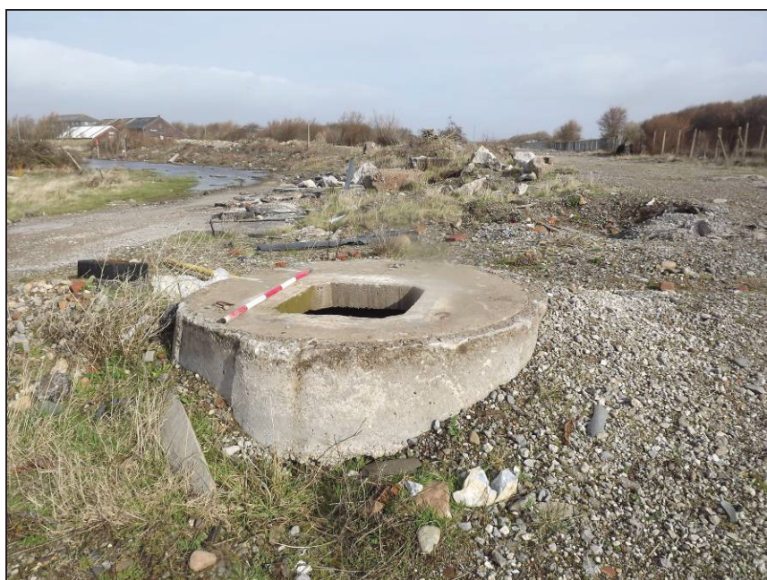
Plate 8: Access hatch for a service run, east side of site
