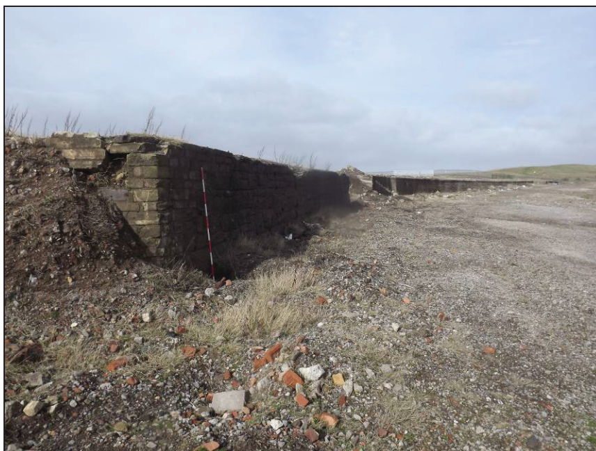
Plate 6: View looking north-west showing the surviving section of retaining wall along the western side of the site
