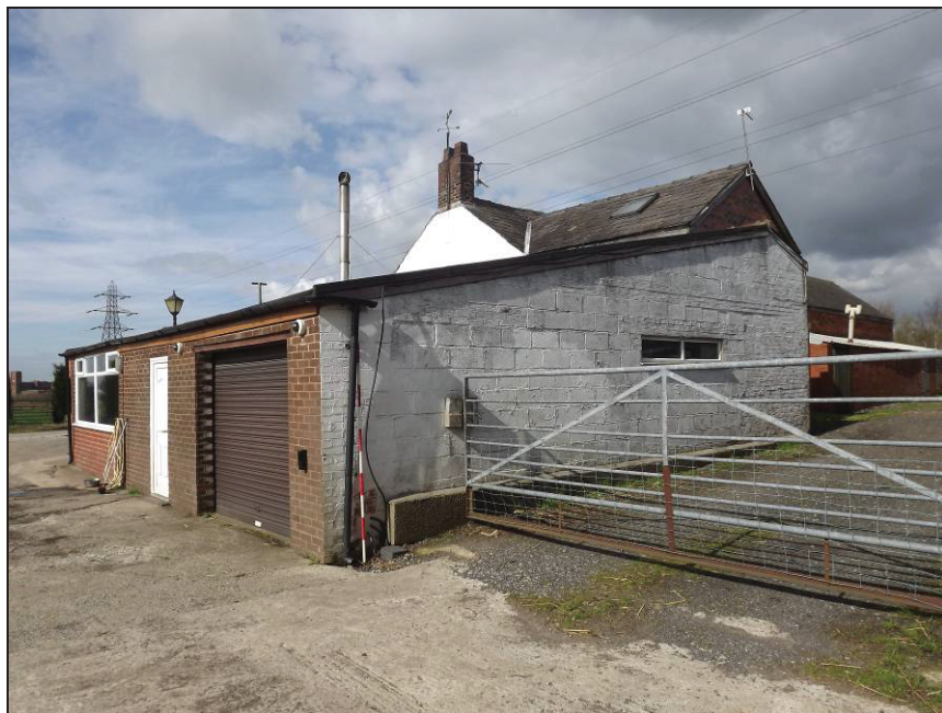
Plate 27: Modern additions at the south end of the north-east and south-east elevations
