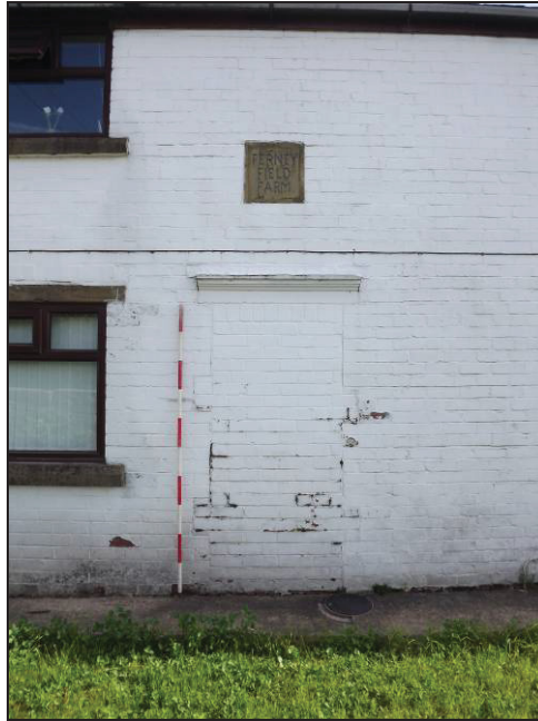
Plate 16: Blocked doorway and modern inscribed stone, south-west elevation (Scale = 2m)
