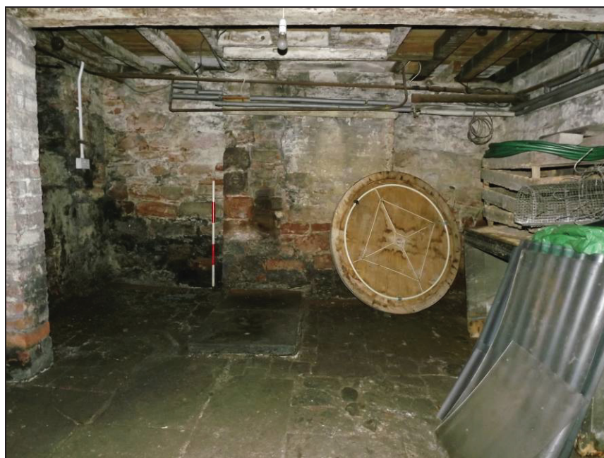
Plate 90: East wall of the cellar showing masonry walls and projecting support for fireplace in kitchen (Room 5) above (Scale = 1m)
