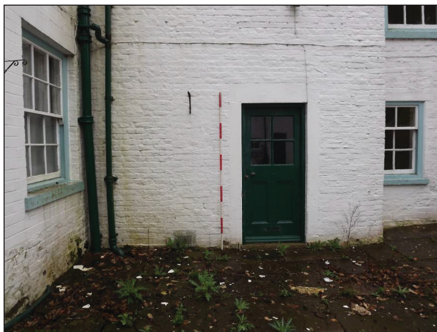
Plate 24: Detail of vertical construction break to left of doorway, western wing (east elevation)
