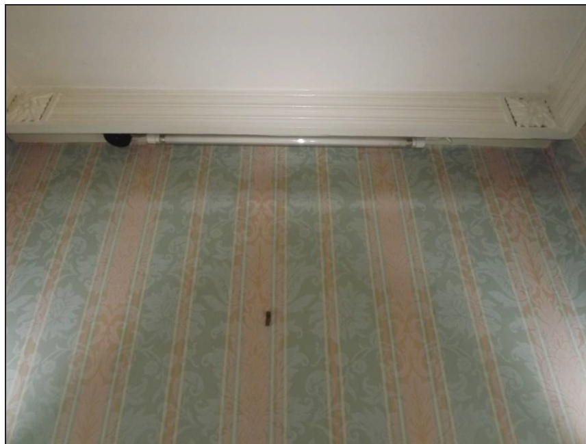
Plate 83: Detail of coving fixed away from the south wall to accommodate strip lights, Room 23
