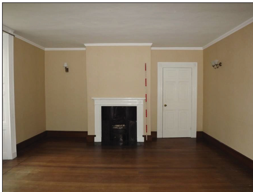
Plate 27: Fireplace in west wall of Room 1, with door to Room 3 to right-hand side
