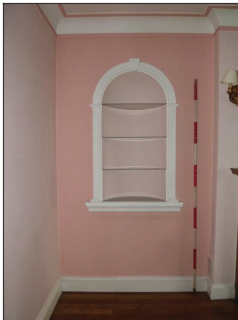
Plate 36: Detail of one of the niches in the east wall of Room 2
