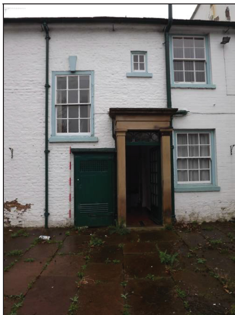
Plate 18: Detail of main entrance to Mulcaster in north elevation, with cellar (green) door to its left-hand side
