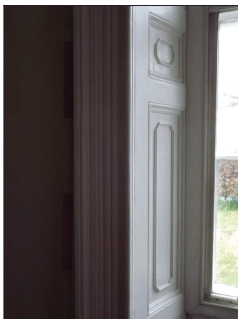
Plate 39: Detail of paneled surround and architrave, window in south wall of Room 3
