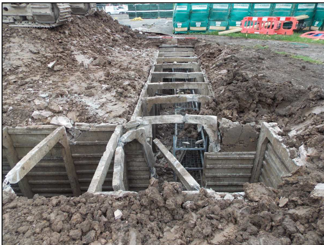
Plate 4: Shot corridors C & E, showing the recess on the right side, looking north
