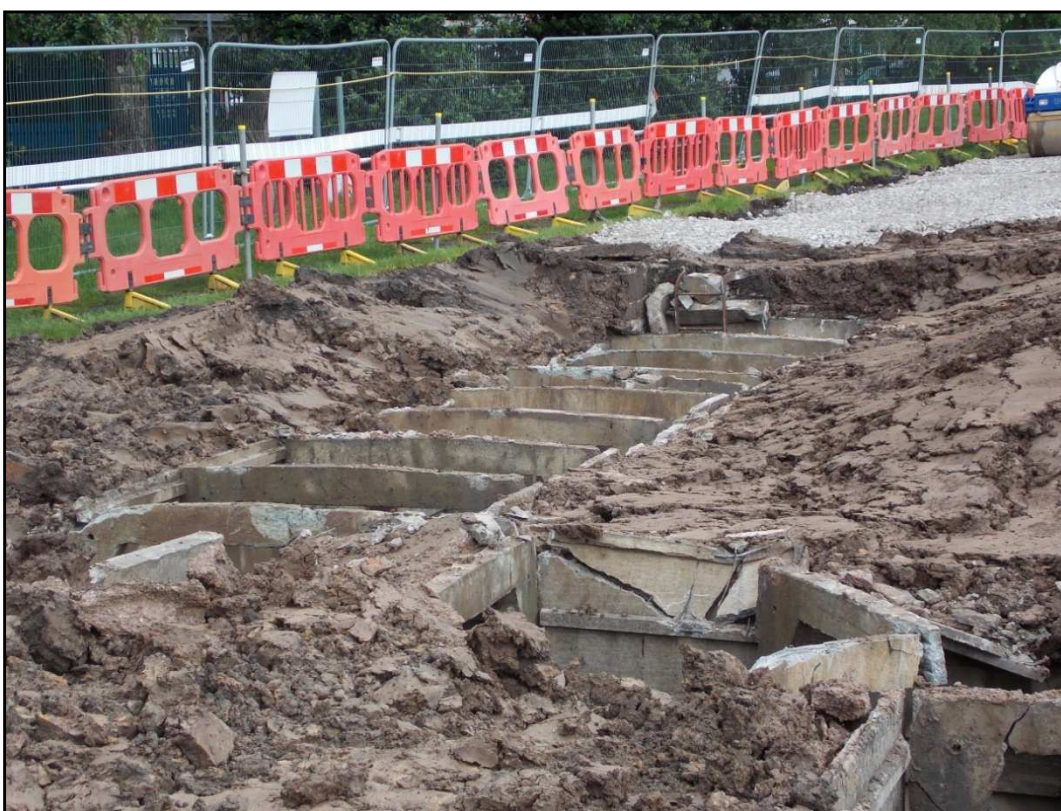
Plate 8: Shot of corridor D, showing escape hatch {110} with ladder in the background, looking northwest
