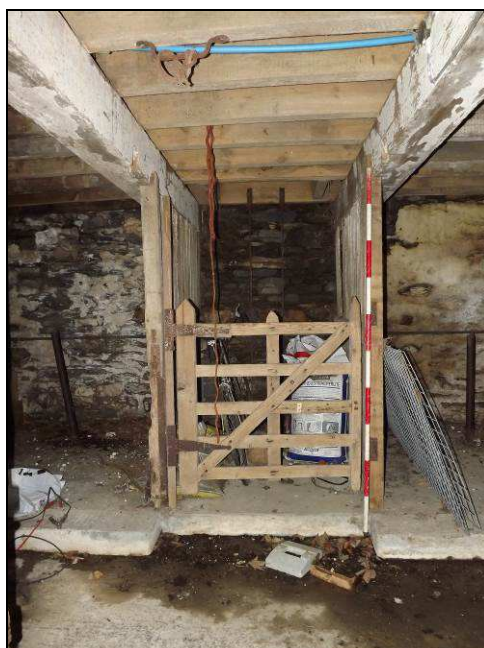
Plate 52: Detail of ladder to first floor, interior of shippon, Building B (Scale = 2m)
