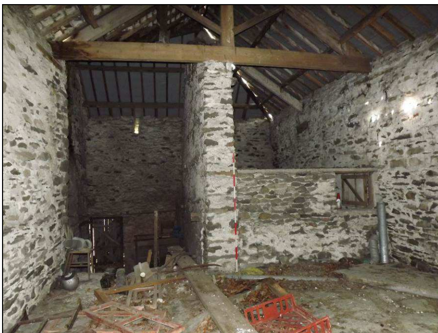
Plate 39: View looking south west from the upper barn showing the spaces over the coal store and the workshop, Building A
