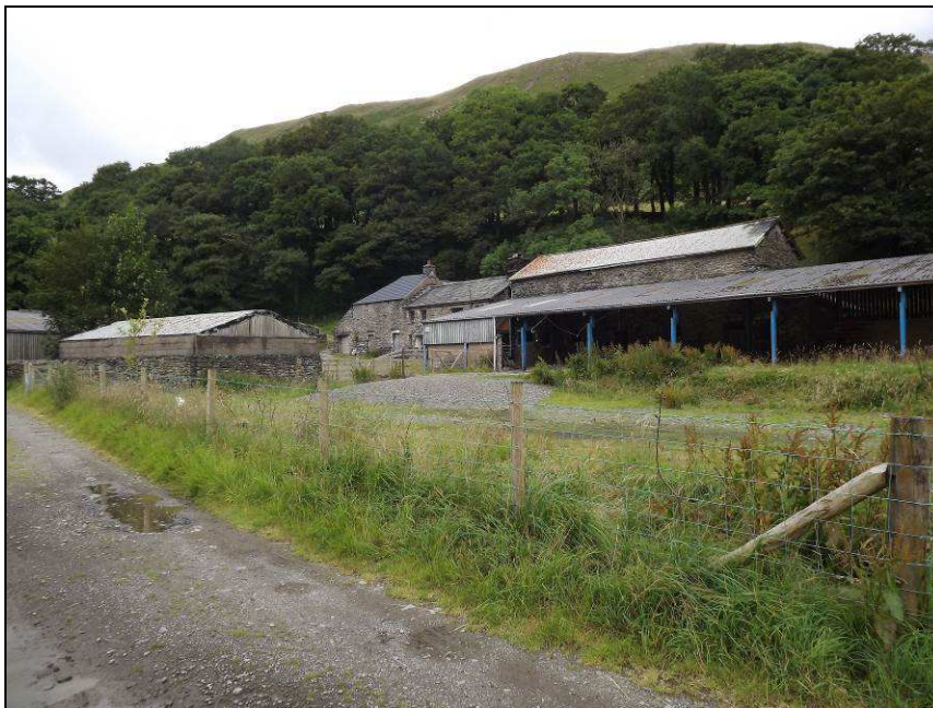
Plate 41: View of Low Borrowdale Farm from the south showing the corrugated sheet roof of Building B to the right of the house
