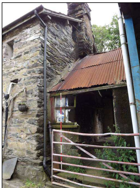
Plate 9: South-east gable of house showing attic window to left of the projecting chimney stack
