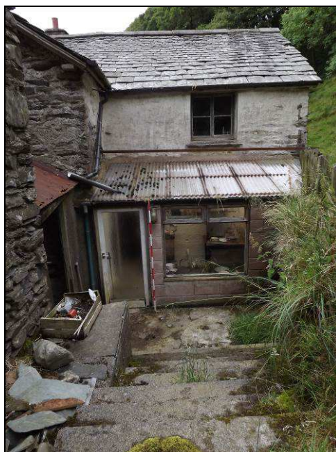
Plate 10: View looking north-west showing the modern conservatory against the north-east elevation of the house
