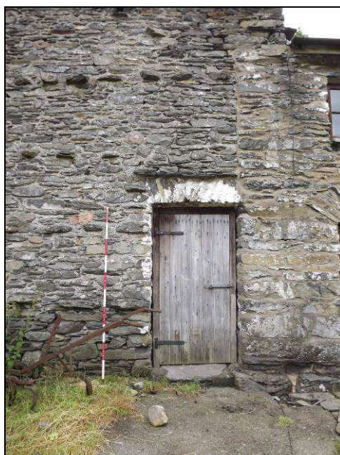
Plate 32: Detail of one of the doorways in the south-west elevation of Building A (Scale = 2m)
