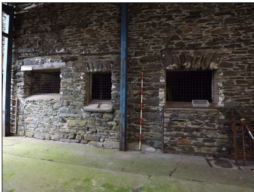
Plate 44: South-west elevation of Building B showing former doorways (now converted to windows) and an inserted window (Scale = 2m)
