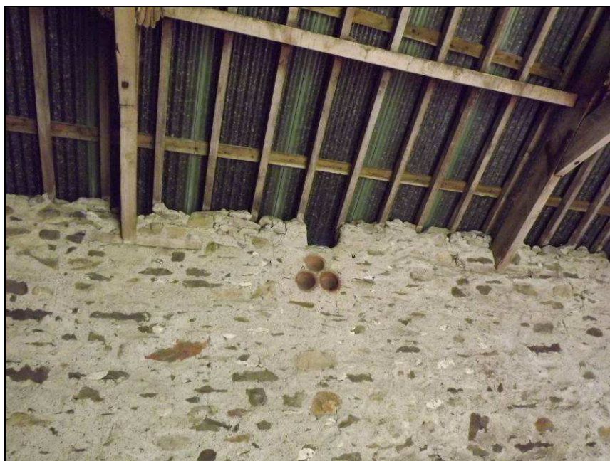
Plate 55: Detail of redundant housing for a roof truss and ceramic pipe ventilation, Building B
