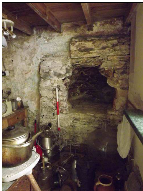
Plate 23: Detail of bread oven in north-east corner of the kitchen (Scale = 1m)
